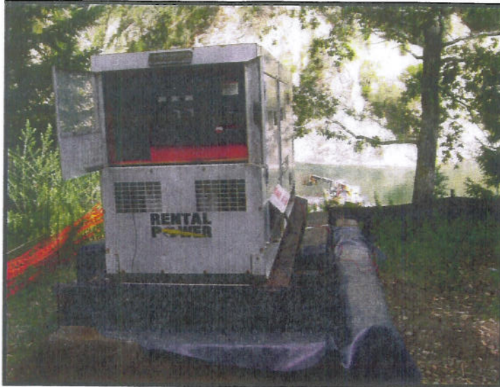
Figure 5: Generator Power Source
