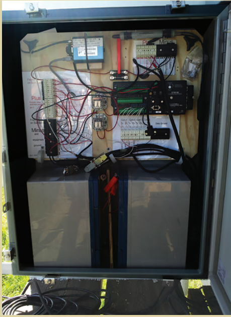
Figure 5. Electronics inside a flow-station gage house.
