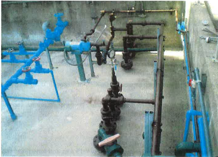
Photograph 5. Gage/data logger in SJWD chemical feed vault
