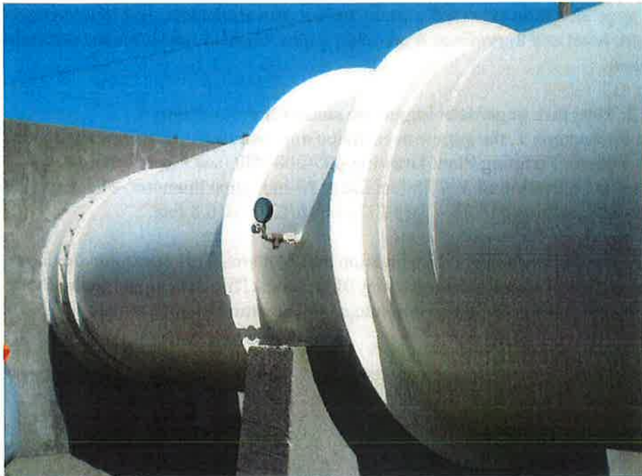
Photograph 2. Gage/data logger on North Fork Pipeline at Hinkle Y
