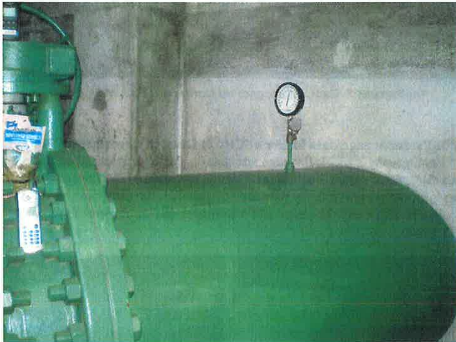
Photograph 1. Gage/data logger on Pump 6 suction pipe
