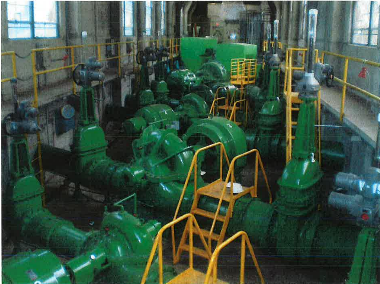
Figure 2-7 Folsom Pumping Plant Pumps, Looking South from Entrance Nearest Dam
