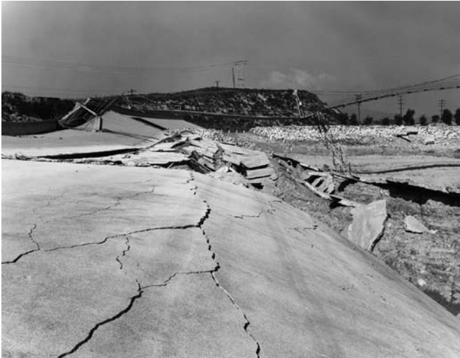
Earthquake damage – Sylmar [February 9, 1971]. Source: DWR
