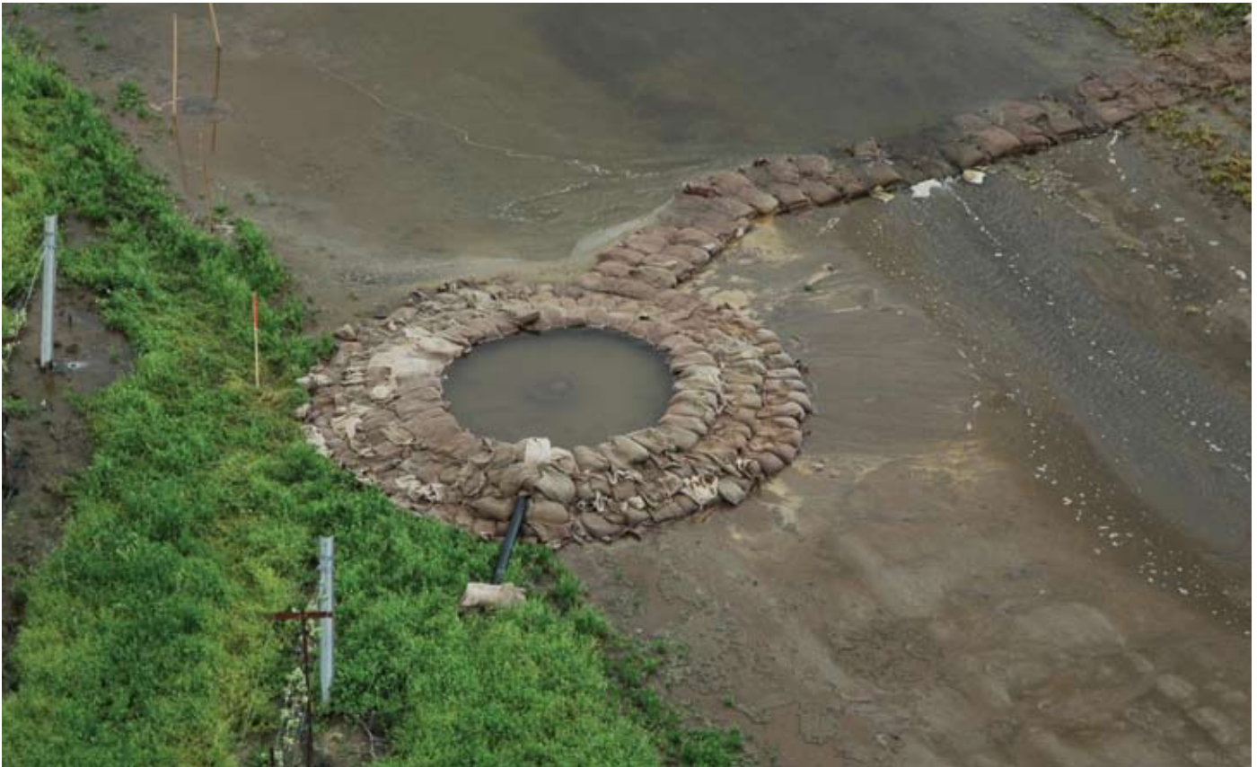
Sandbags temporarily control a sand boil on Staten Island on June 18, 2007. The muddy water indicates that material in the levee or its foundation is being washed away. Unnoticed, sand boils can lead to a failure of the levee. Source: DWR
