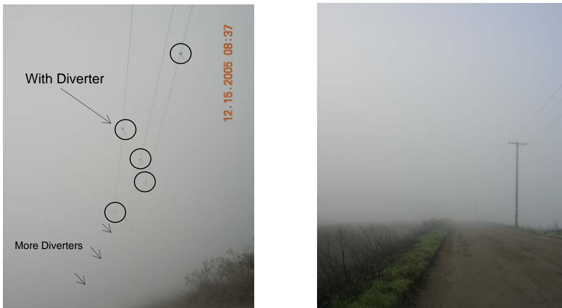
Figure 2. Distribution power lines at the study site (Staten Island, Walnut Grove, California). Heavy winter fog reduces visibility of distribution power lines with (left) and without (right) aerial marking devices. These devices, designed to increase line visibility, may not be effective in heavy fog.
