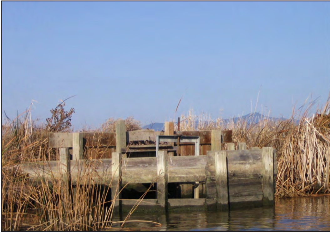
Photo 3. This photo depicts an outfall structure that is common to the project area.
