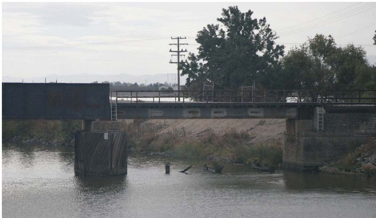
Figure 2. Railroad bridge located upstream of the RWCF. Note the bridge supports and remnant supports underneath the bridge, which provide holding habitat for piscivorous fish.
