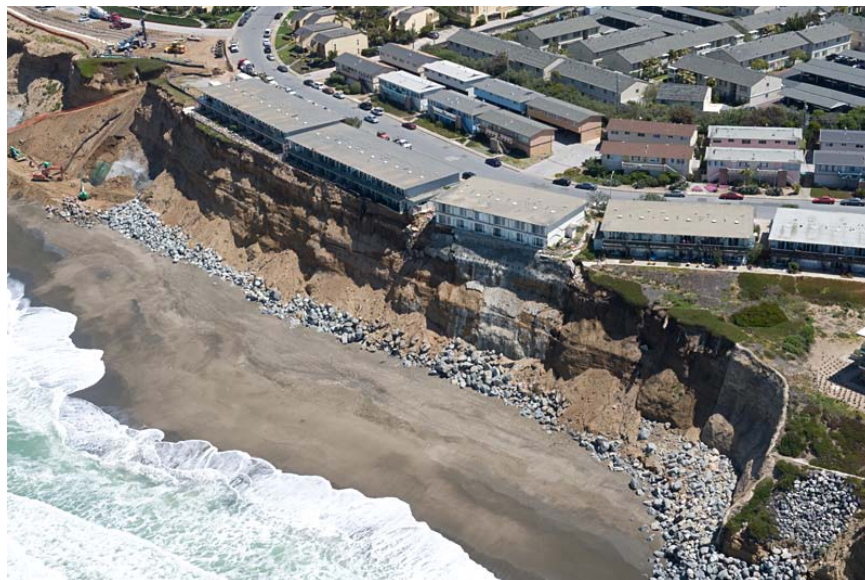
FIGURE 6.3 Erosion of poorly consolidated sedimentary cliffs at Pacifica, south of San Francisco, is threatening these apartments, and residents have had to move out. Riprap protection has been placed at the toe of the bluff in an attempt to slow the erosion. SOURCE: Hawkeye Photography.
