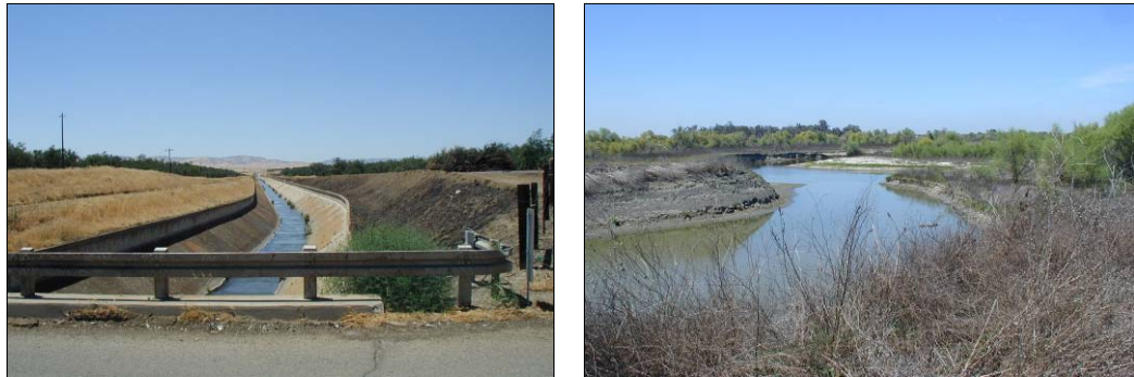
Photograph 2.2.1-2. Newman Wasteway at DMC (left) and at San Joaquin River Terminus (right)
