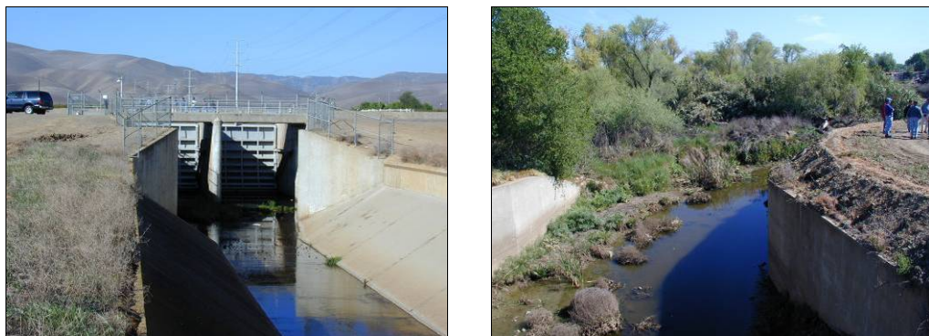
Photograph 2.2.1-3. Westley Wasteway at DMC (left) and at Bypass to Private Refuge (right)
