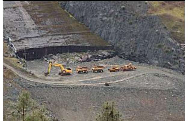
Ben Furtado/Journal File The concrete work that was part of the original dam construction project in the 1960s and 1970s can be seen above heavy equipment used as part of work now taking place in the American River canyon to restore the river channel.
