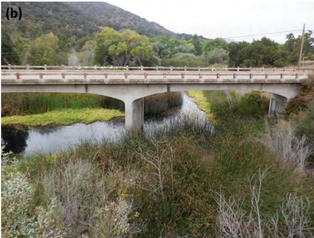
Figure 56: Photo points (M-6) collected at Highway 154 Bridge looking downstream in (a) September 2005 and (b) September 2021.
