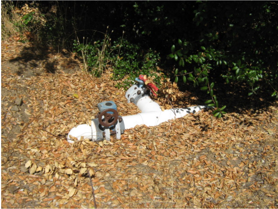
RESERVOIR #2 OUTLET PIPE & GRAVITY DIVERSION WORKS FOR VINEYARD IRRIGATION
