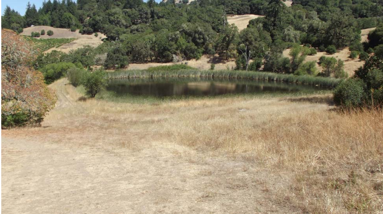
Figure 7: Reservoir 2 facing north-west. The dam can be seen on the left and far sides of the reservoir.
