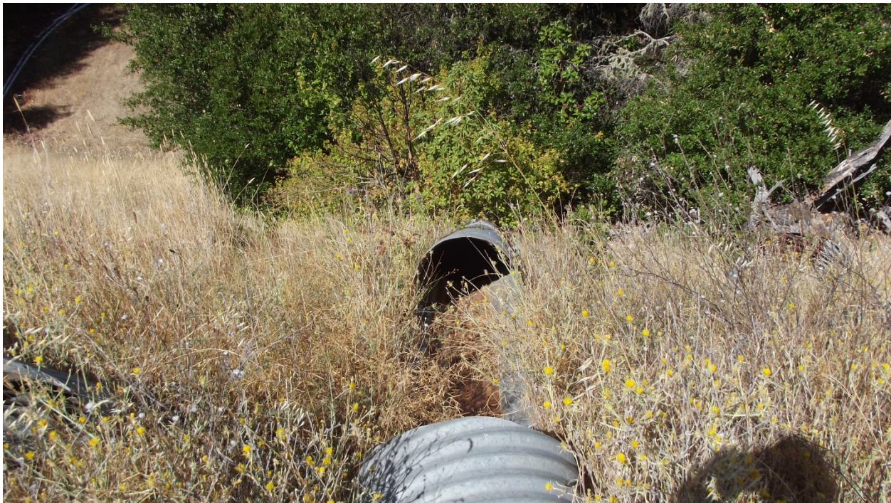
Figure 4: Spillway pipe leading down the face of the dam to the stream connecting the reservoirs.
