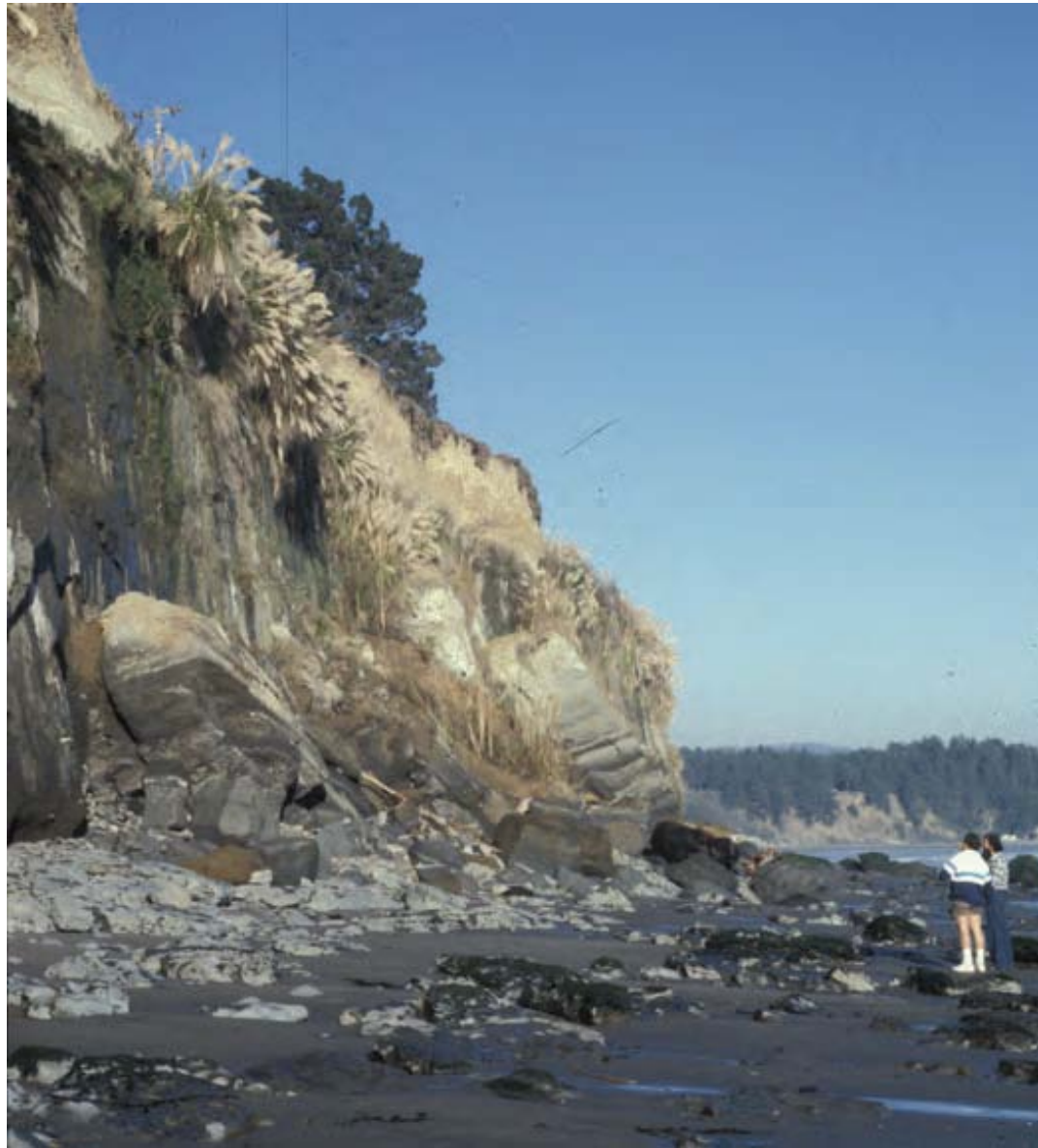
Figure 16: Block failure along joint sets accelerated by seepage in sedimentary rocks of northern Monterey Bay, California. Seepage imparts a dark shade to the cliff, visible at left side of photo. Note pampas grass in area of seepage. From Figure 26 of Hampton, M.A., and others, USGS Professional Paper 1693, 2004.
