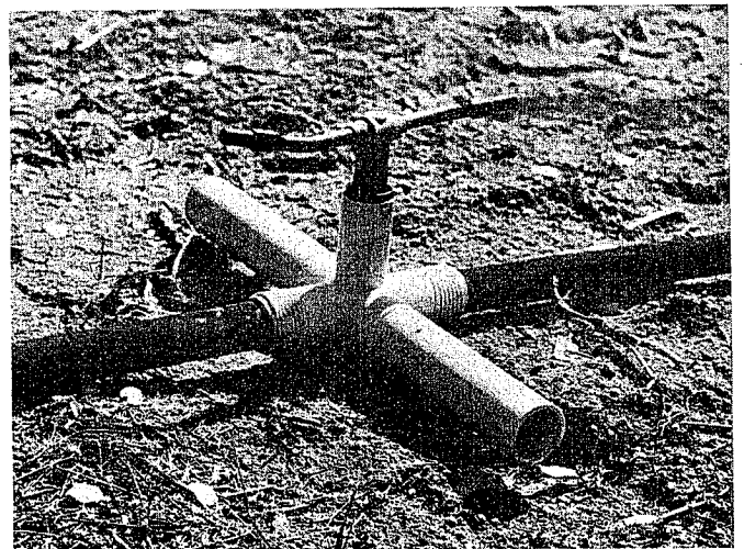
An under-tree sprinkler.
