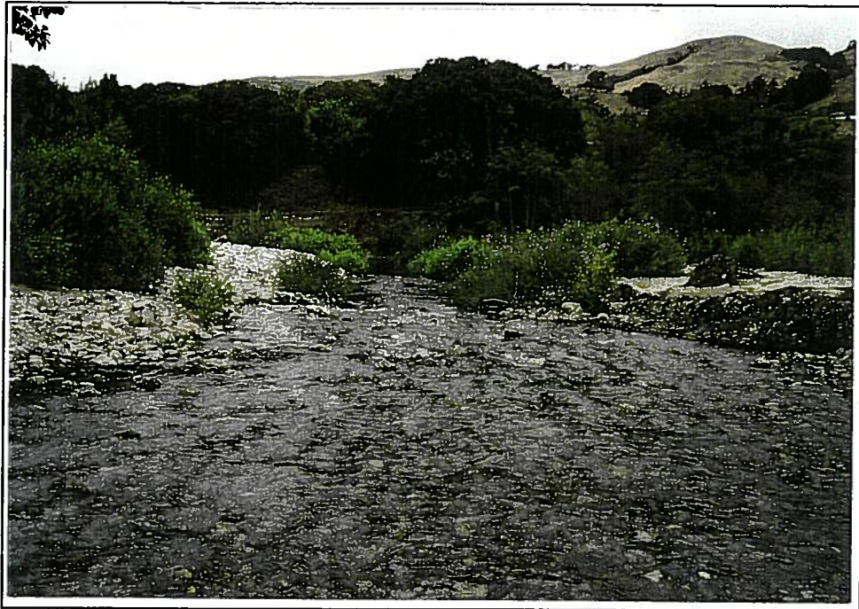
Plate 1. View downstream of Big Sur River from footbridge across Big Sur River near parking lot in Andrew Molera State Park. The remains of gabion revetments are located on the right side of the channel.
