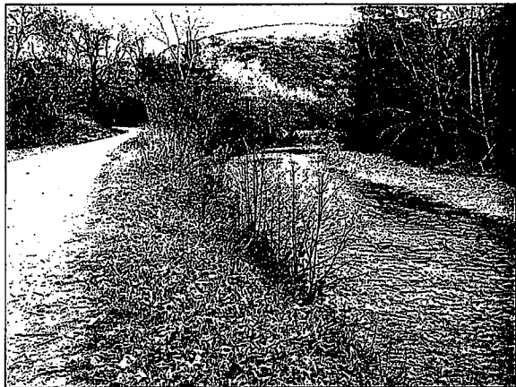
1997-98 Right bank failure at ranch road. (RM 1.29-1.32). Note alder and willow recruitment at toe. Road realignment and bio-engineered slope treatment proposed.
