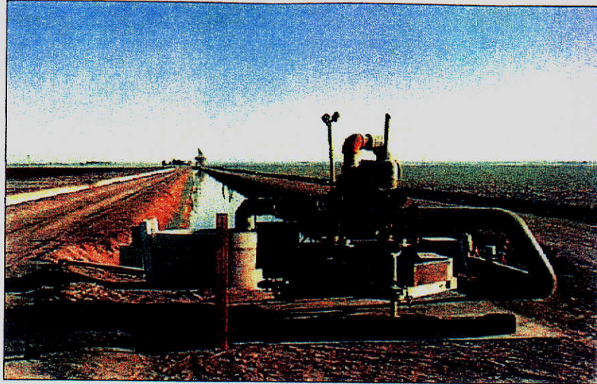
Permanent Tailwater Return System and Pond
