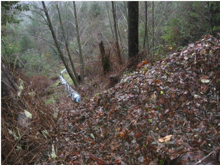
Photo 16 – 14-inch diameter penstock pipe.
