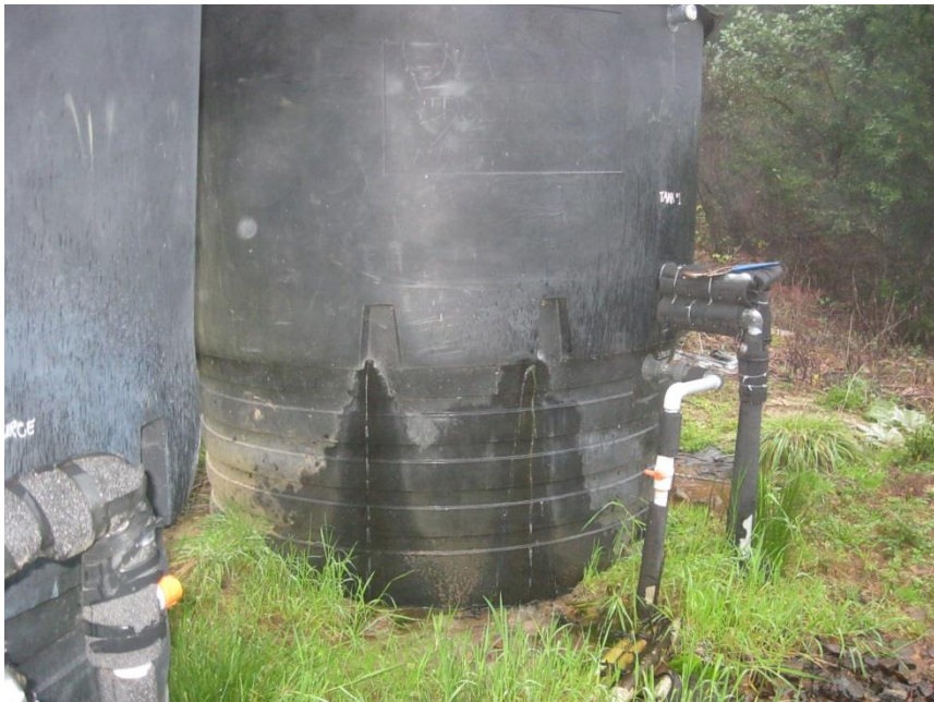
Photo 14 – leaks coming from one of the 3,000 gallon water tanks used for filtration.
