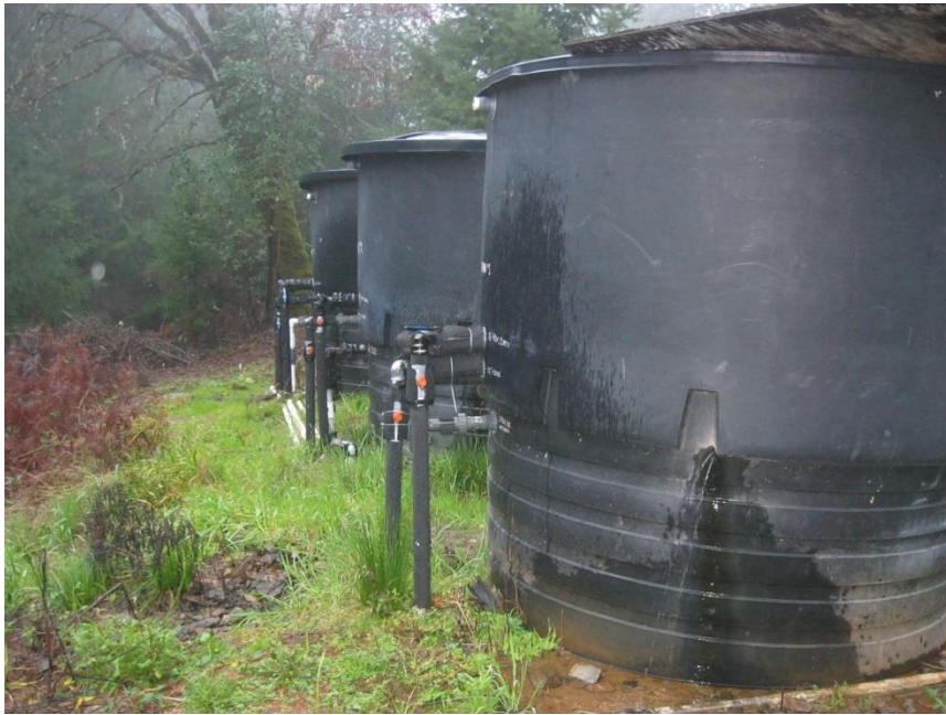
Photo 13 – (3) 3,000 gallon storage tanks.
