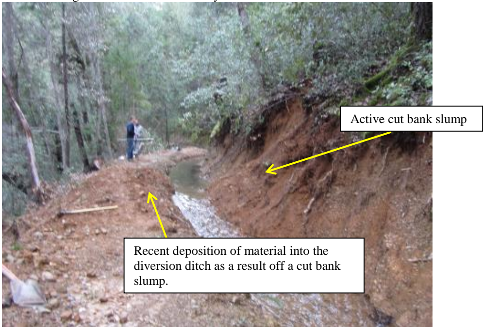
Photo 8 – Area of active cut bank slumping.
