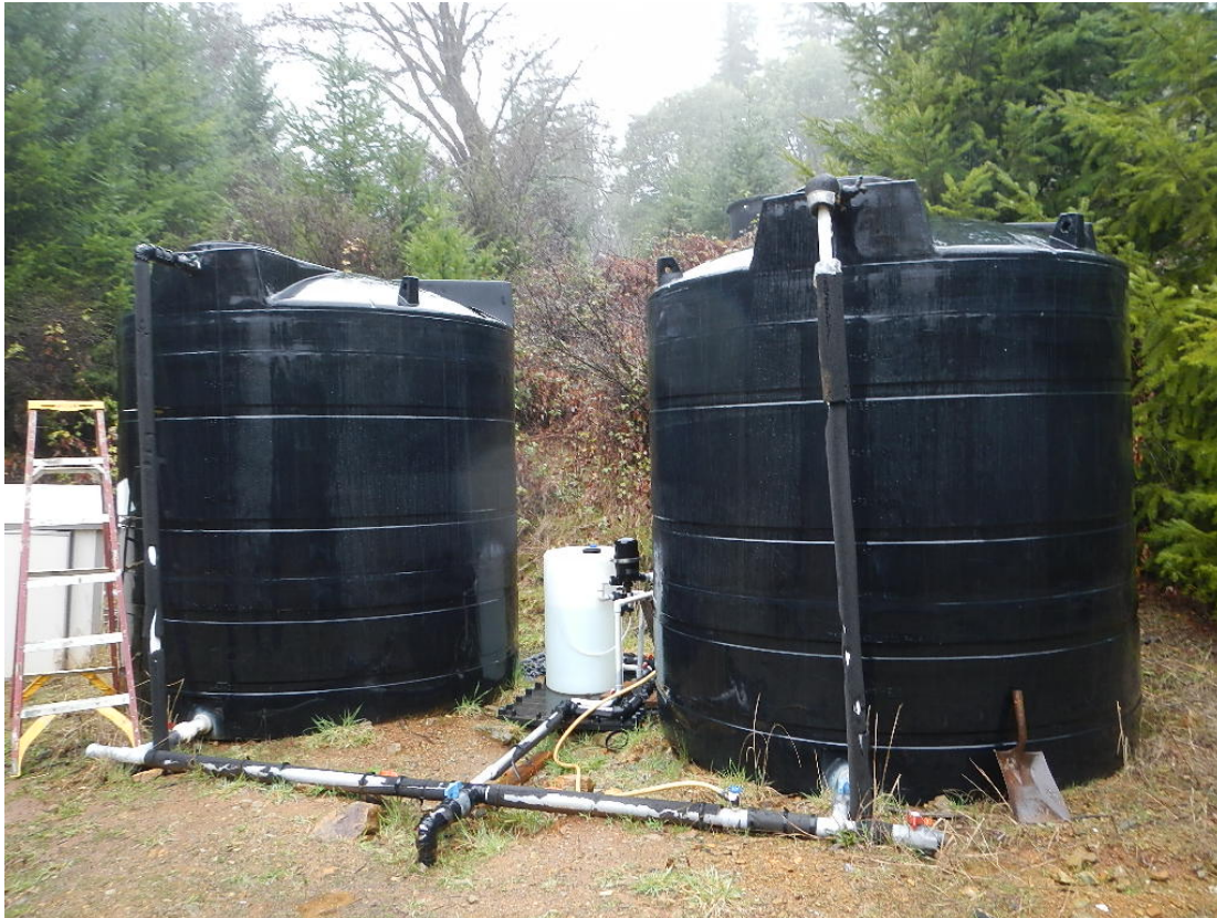
Figure 3. Domestic water treatment facility
