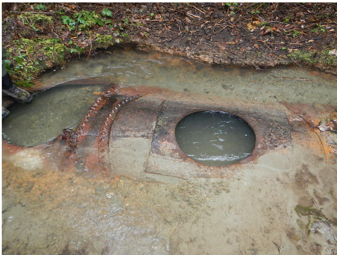
Figure 6. Failed Sediment Trap
