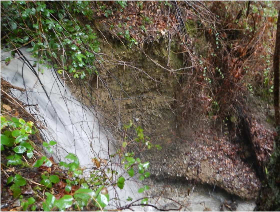
Figure 9. Gully headcut (approx. 15 feet deep) where MMR ditch leaves MMR into Irving Creek drainage.
