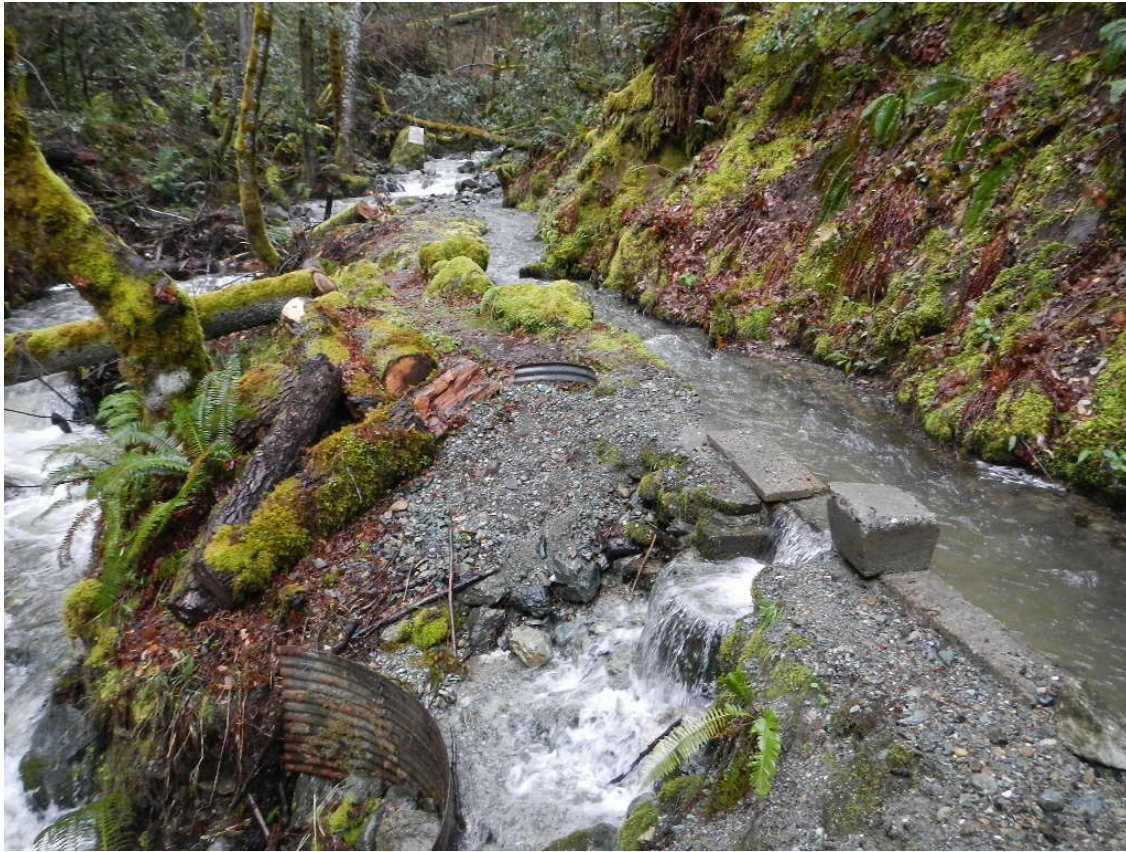
Figure 7. MMR ditch overflow just below Point of Diversion (POD).
