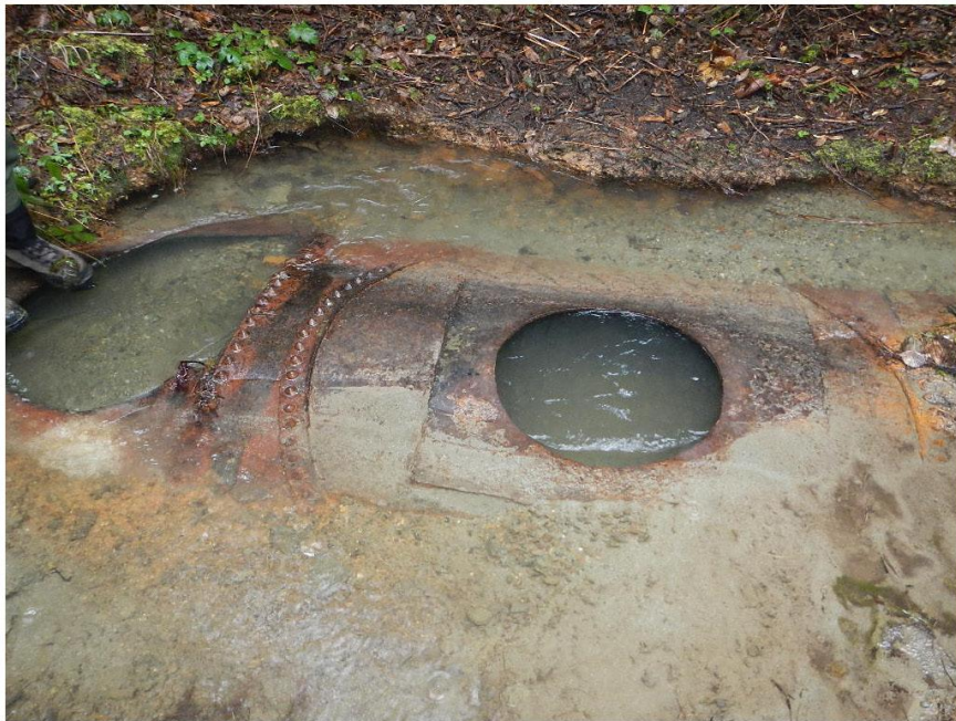
Figure 6. Failed Sediment Trap
