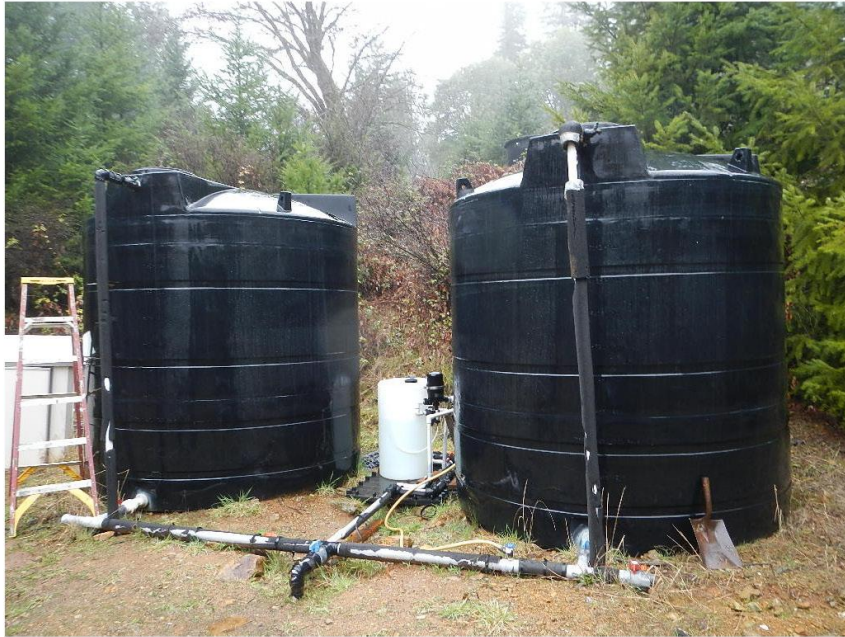
Figure 3. Domestic water treatment facility
