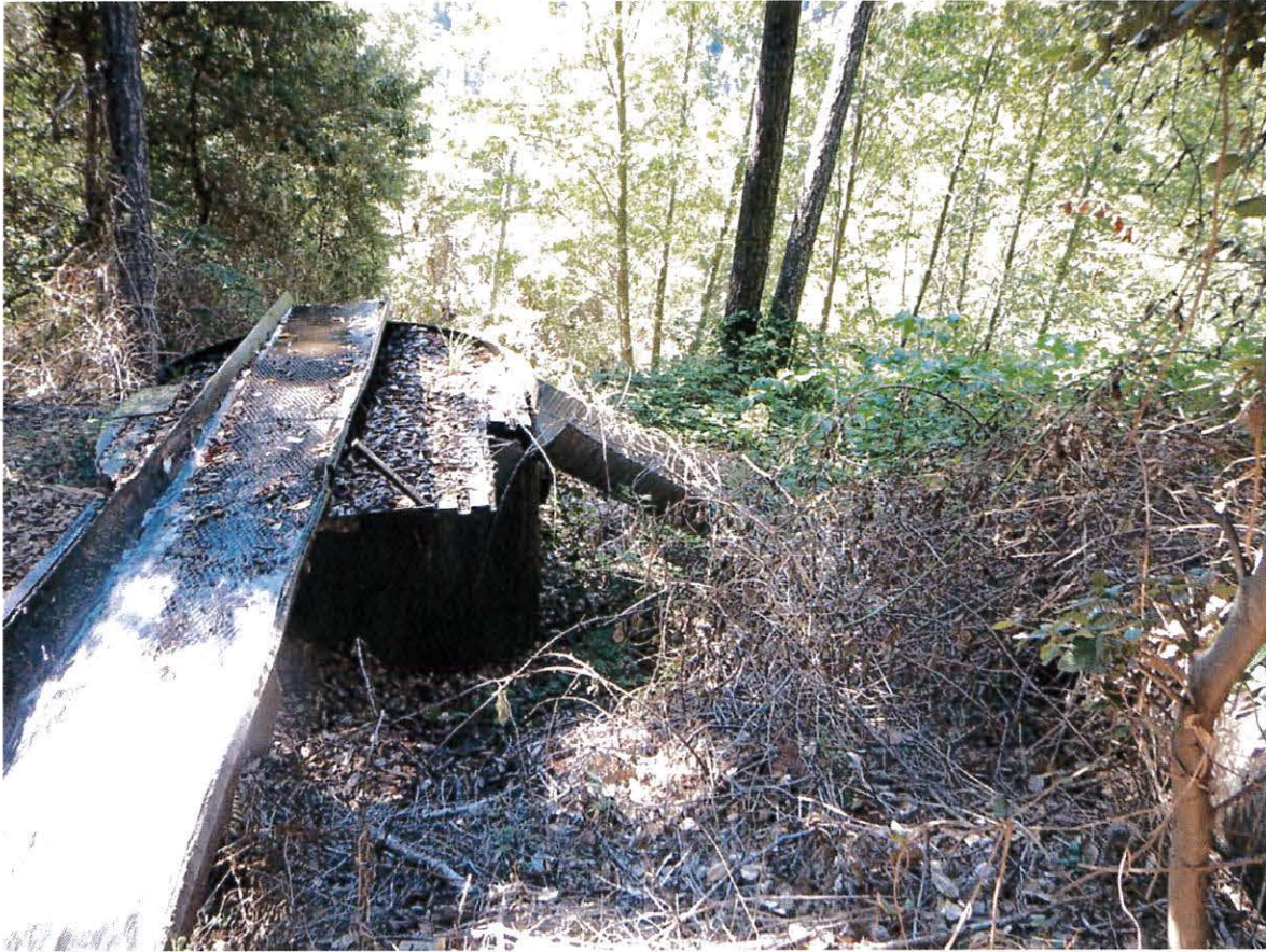
Photograph 7. Forebay to pressurized system. Flows enter system through the screen in the half pipe section.
