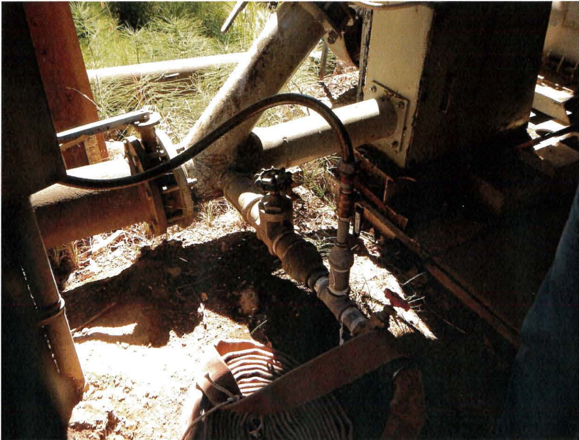
Photograph 5. Junction near hydro-power unit. Large diameter pipes convey water to Pelton wheel. Small diameter pipe that tees at a 90 degree angle conveys water to heat sink resistor and hose.
