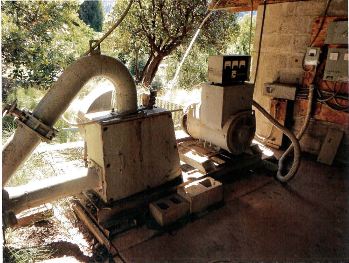
Photograph 4. Micro-hydro power plant diversion flows enter from the pipes on the left of the photograph. Heated effluent from the heat sink resistor is visible near the top of the photograph near the roof beam.
