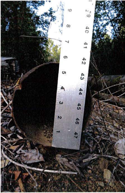
Photograph 3. Pipe adjacent to 14" Pipe. End of pipe was crimped making estimation of Interior diameter imprecise.
