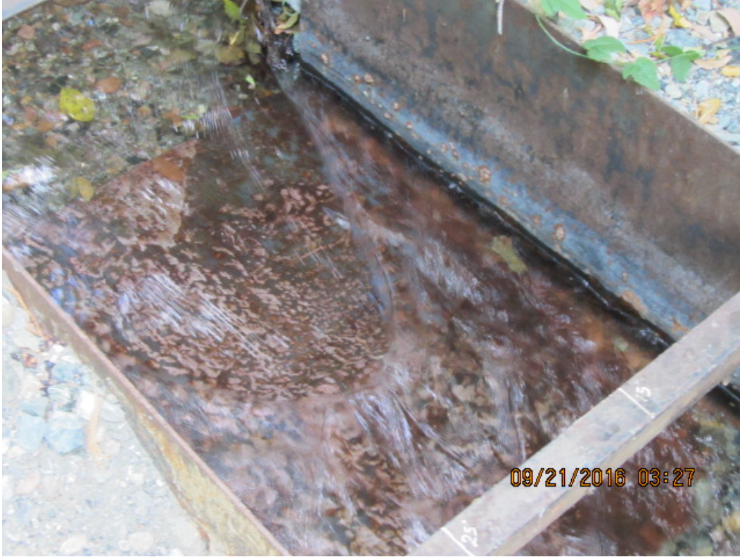
Exhibit MMR-02, Photograph #6 showing a culverted portion of the diversion on September 21, 2016
