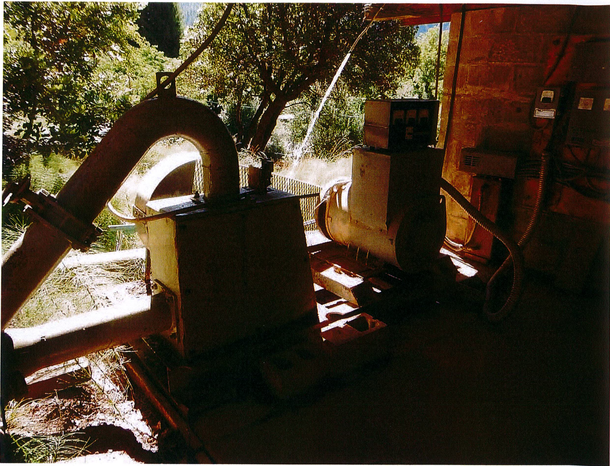
Photograph 4. Micro-hydro power plant diversion flows enter from the pipes on the left of the photograph. Heated effluent from the heat sink resistor is visible near the top of the photograph near the roof beam.
