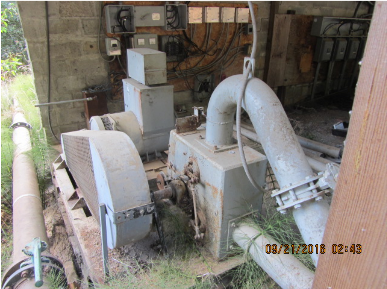
Exhibit MMR-04 Photograph #1 – The hydroelectric powerplant in September 2016
