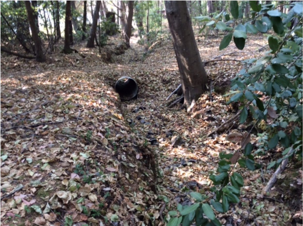
Exhibit MMR-06 Photograph #1 – End of Marble Mountain Ranch return flow channel to Irving Creek outfall showing no flow present in spring 2017
