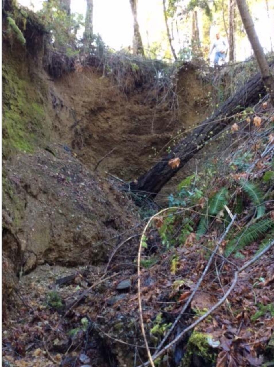
Exhibit MMR-06 Photograph #2 – Headcut of Irving Creek outfall showing no flow present in spring 2017
