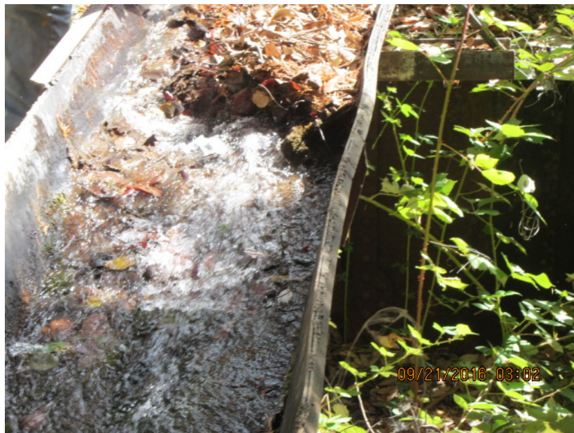
Exhibit MMR-08 Photograph #2 – a culverted portion of the diversion just before the water meets the screened portion of the diversion
