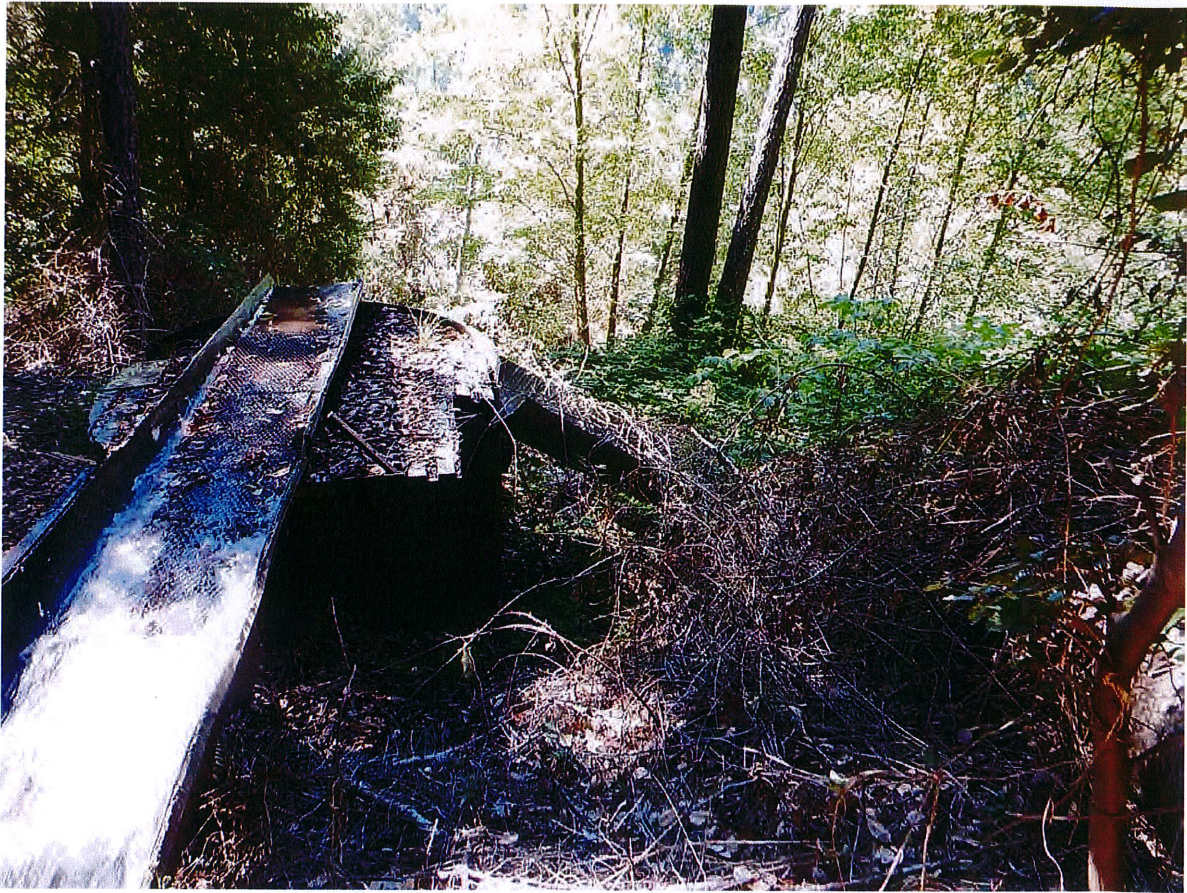
Photograph 7. Forebay to pressurized system. Flows enter system through the screen in the half pipe section.
