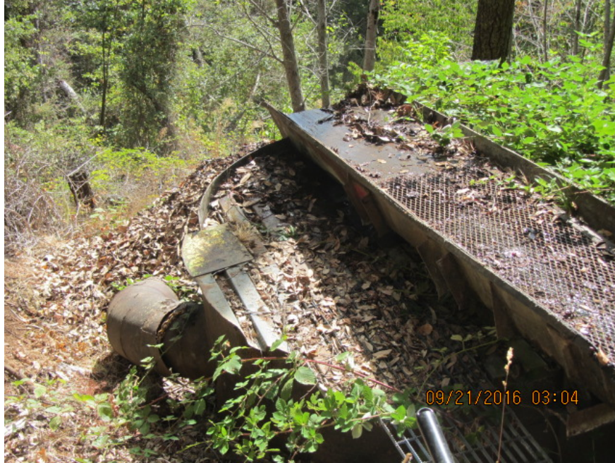
Exhibit MMR-08 Photograph #1 – screened portion of diversion and culvert before water in the diversion moves to treatment and hydroelectric systems
