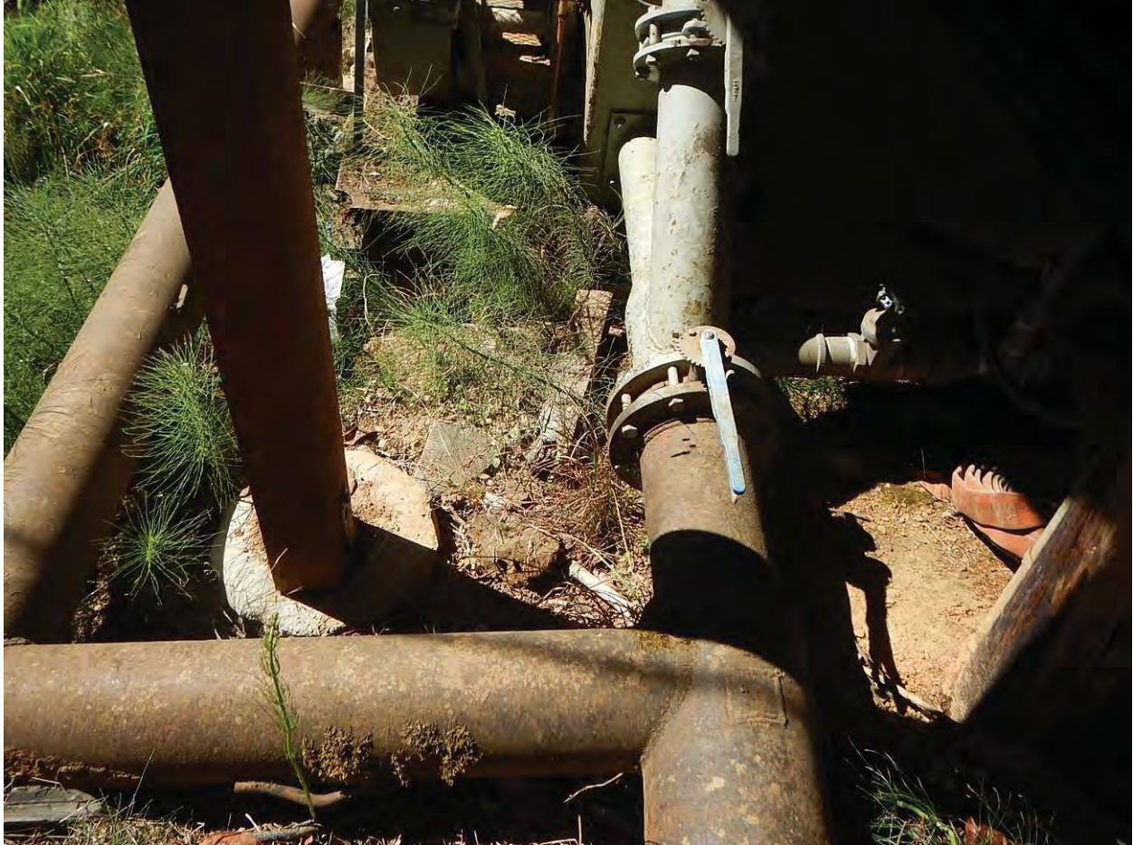
Photograph 6. Junctions near power plant. Tee near the bottom of the photograph serves as junction for flow to power plant and irrigation system. Flow conveyed into the pipe to the left of the photograph serves the irrigation system.
