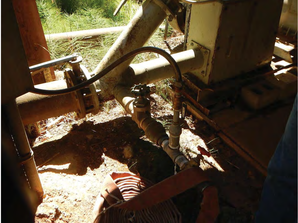
Photograph 5. Junction near hydro-power unit. Large diameter pipes convey water to Pelton wheel. Small diameter pipe that tees at a 90 degree angle conveys water to heat sink resistor and hose.
