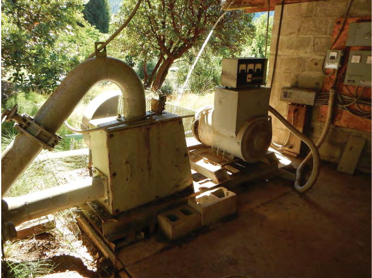
Photograph 4. Micro-hydro power plant diversion flows enter from the pipes on the left of the photograph. Heated effluent from the heat sink resistor is visible near the top of the photograph near the roof beam.
