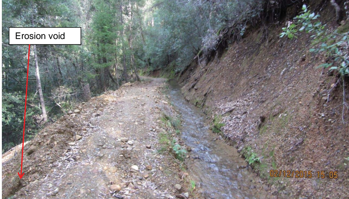
Image 21- Point 14, a cut bank that appears to have slumped in the recent past, causing water to overtop the berm and erode the berm and lower slopes. (Photo 8520 and 8521 composite)
