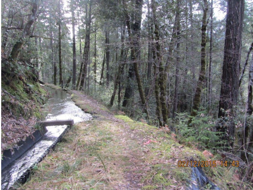
Image 13- point 7, shows the end of the flume in the previous photo; note the black plastic sheeting on the outboard slope face, and the low outboard berm as the diversion ditch exits the flume. The lack of freeboard creates a high potential for overtopping and erosion. The presence of the pipe section and plastic sheeting in the area suggests that the berm or underlying slope in this area has likely failed in the past. (Photo 8483)
