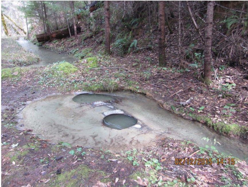
Image 8- at Point 3, shows a closer view of the buried tank car with stored sediments visible. (Photo 8450)
