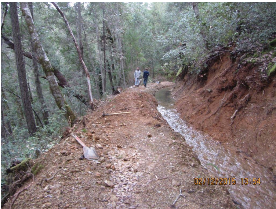
Image 24- Point 17 shows a segment of channel with an active cut bank slump and evidence of recent repairs to the outboard berm.
