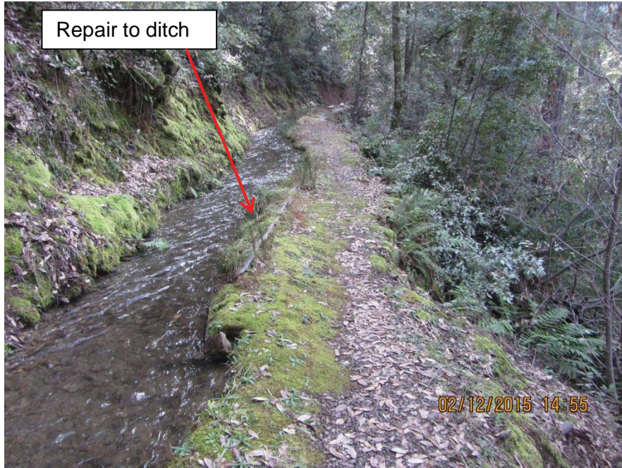
Image 17- Point 11 is another 150-200 feet of ditch with a low freeboard and evidence of past failures; this ditch segment leads to a section of ditch subject to a recent bank failure. I observed erosion scars on the lower slopes that are now overgrown with ferns and small shrubs. (Photo 8499)
