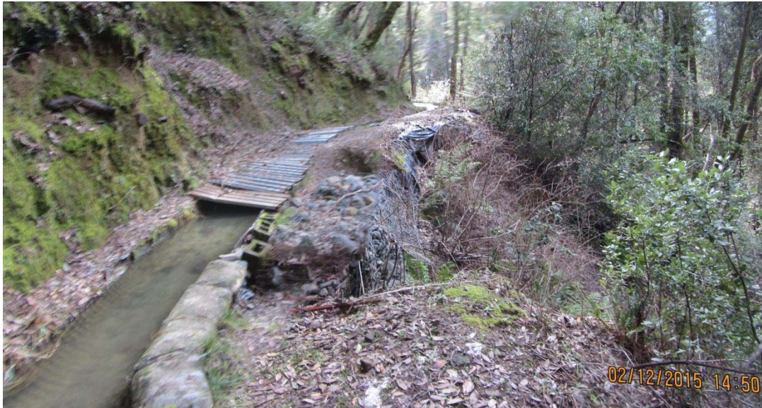
Image 15- shows Point 9, a significant failure point, likely caused by a cut bank slump filling the diversion channel and diverting the stream flow. Note the cut bank slump above and the erosion void downslope. This failure likely accelerated erosion on lower slopes and into the nearby streams. (Photo 8490 and 8491 composite)
