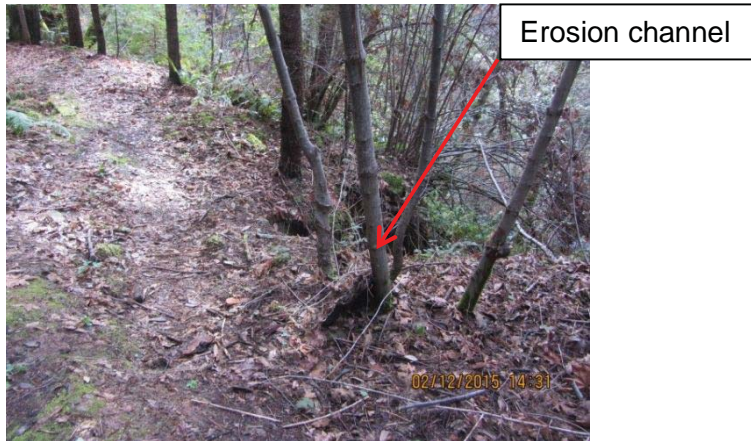
Image 6- shows the erosion channel downslope of Point 3.
