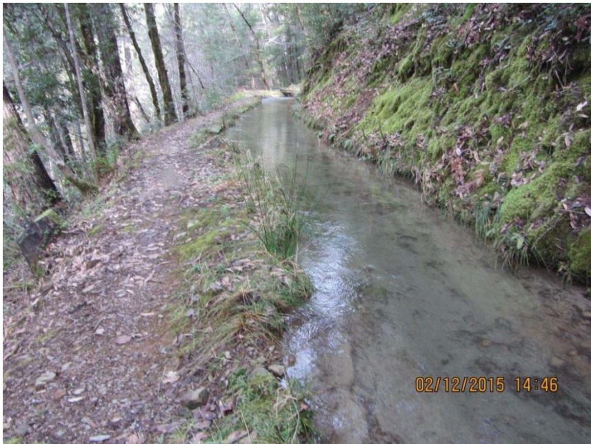
Image 14- shows point 8, an approximately 150-foot section of the channel downstream of Point 7, where the low berm and full ditch likely creates a high potential for berm or slope failure, erosion, and sediment transport downslope. I observed concrete blocks at various locations along the outboard edge of the berm throughout this segment, likely to rebuild or reinforce berm sections. (Photo 8486)
