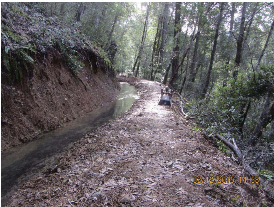
Image 20- Point 13 shows a large continuous cut bank slump that extends for approximately 220 feet. Based on my observations, it appears the cut bank slumped along this stretch over this past winter, delivering approximately 10 yds 3 of sediment into the ditch, blocking the channel, and causing water to overtop the berm
