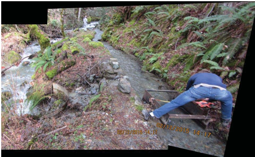
Image 4- shows Point 2, a failure along the outboard berm, approximately 70 feet downstream of Point 1, allowing some of the water in the ditch to flow down to Stanshaw Creek, potentially resulting in erosion and sediment transport. This location appears to have failed repeatedly in the past. The instream flume in the Ditch just downstream of this failure is used to measure flows entering the diversion. (Photo 8454 and 8455)
