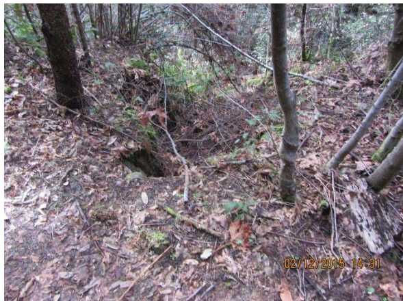
Image 7- shows the erosion channel downslope of Point 3. The void is visible here in the foreground; the erosion extends downslope an unknown distance.
