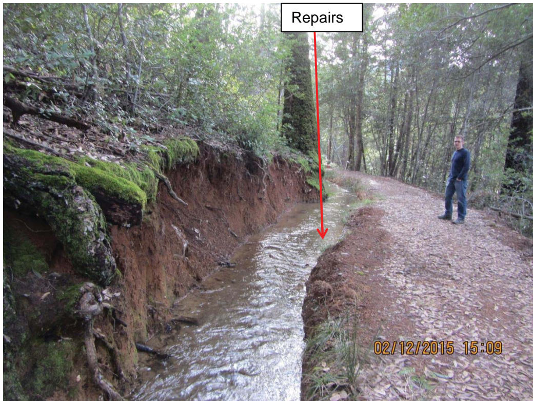
Image 22- Point 15 shows an active cut bank slump, and evidence of recent repairs to the ditch and berm. (Photo 8523)
