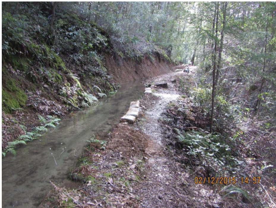
Image 18- Point 12 shows evidence of a recent bank failure that caused water to overtop the outboard berm and erode slopes below the ditch. The outboard ditch shows signs of seepage throughout this length. Note the sand bags and fresh soils along the outboard berm, indicating recent repairs. Also, note the 50-75 foot section of the cut bank with exposed soils. (Photo 8503)
