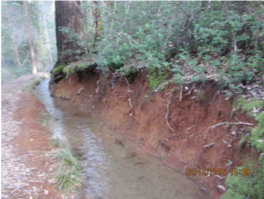
Image 23- Point 16, another cut bank that has a high risk of failure. Note the steep, near vertical slope of this cut bank, which indicates that the bank is still likely to erode. The roots hanging out of the cut bank are indicators of the erosion that has occurred. Most cut banks are originally constructed in a planar form with no visible roots protruding. Over time the cut bank erodes, exposing the roots, and leaving an indicator as to the amount of soil that has eroded or slumped. (Photo 8525)
