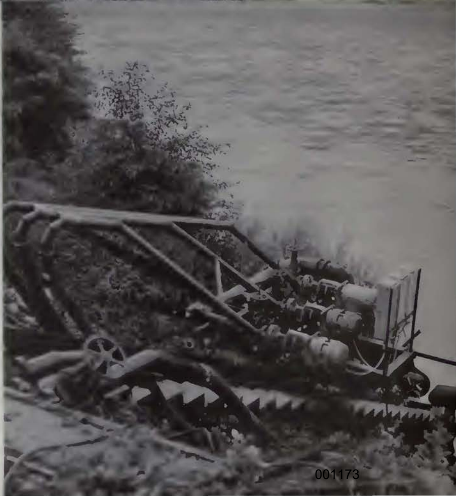
Pumping Installation, Klamath River, Orleans Veneer and Lumber Co.
