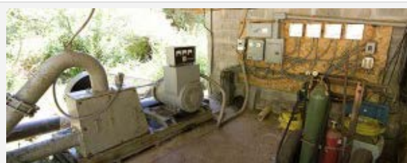
Entirely off the grid, Marble Mountain Ranch generates electricity with the small hydroelectric plant
