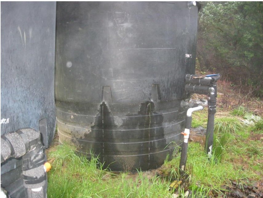
Photo 14 – leaks coming from one of the 3,000 gallon water tanks used for filtration.
