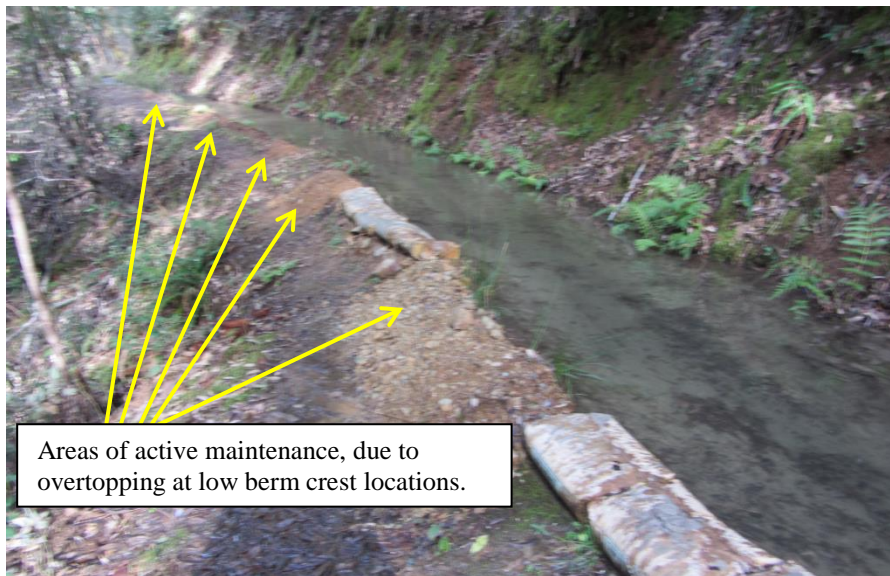
Photo 10 – limited free board space within the ditch.
