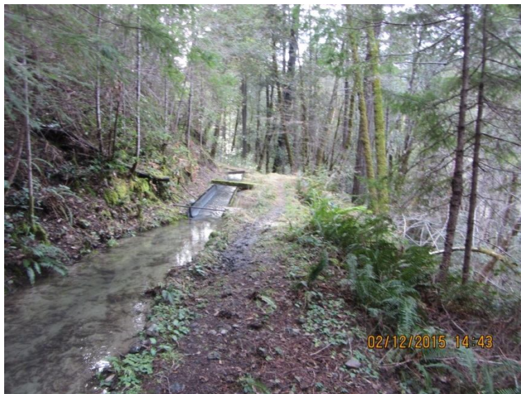
Image 12- shows Point 6, where the diversion channel is full, leaving no freeboard should it rain or the ditch receive a bank slump upstream. It appears the outboard berm may have failed in this area in the past, and at present is seeping, indicating that a portion of the berm may be saturated. Stanshaw Creek is within 200 feet; any failure here likely results in direct delivery of sediment and erosional debris. The flume section visible in the photo appears to have been installed to remedy previous ditch failures and/or to prevent future failures.
