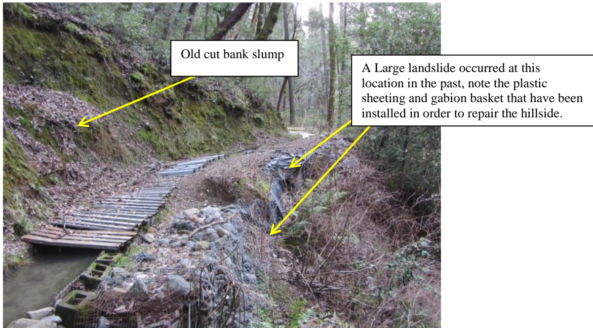
Photo 11 – Large landslide caused by cut bank slump damming ditch and redirecting diverted flow downhill..
