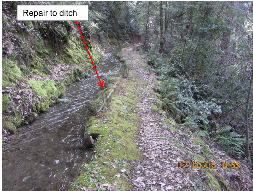
Image 17- Point 11 is another 150-200 feet of ditch with a low freeboard and evidence of past failures; this ditch segment leads to a section of ditch subject to a recent bank failure. I observed erosion scars on the lower slopes that are now overgrown with ferns and small shrubs. (Photo 8499)
