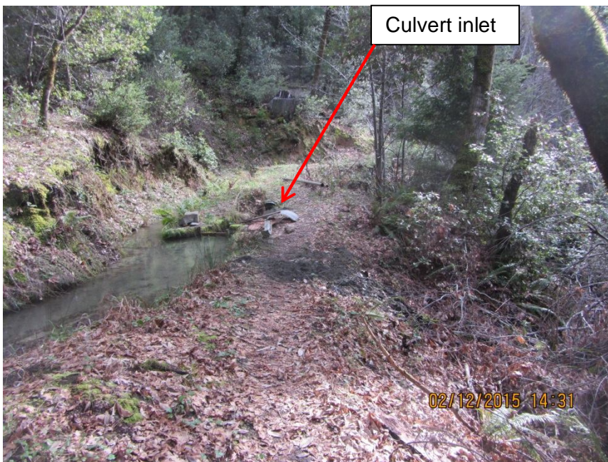
Image 9- at Point 4, shows the partial diversion of the ditch into an unnamed tributary to Stanshaw Creek through the inlet of a 12-inch culvert, before the diversion ditch is routed across the stream in a lined ditch. The culvert is shotgunned, which appears to have caused significant instream erosion in the downslope channel. The stream above the crossing is 3-4 feet wide at bankfull width; the eroded stream channel below the diversion crossing is 12-14 feet wide, and does not appear stable. At this location, I also observed muddy soils in the berm adjacent to the ditch, indicating that seepage from the ditch is saturating surrounding soils, which may lead to catastrophic failure of the ditch. (Photo 8441)
