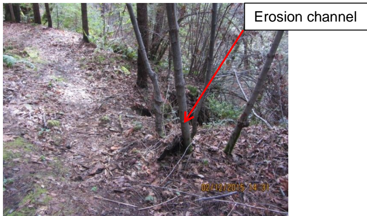
Image 6- shows the erosion channel downslope of Point 3.
