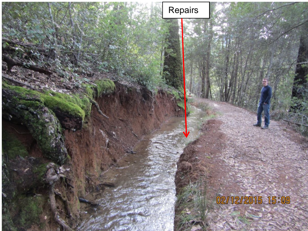
Image 22- Point 15 shows an active cut bank slump, and evidence of recent repairs to the ditch and berm. (Photo 8523)
