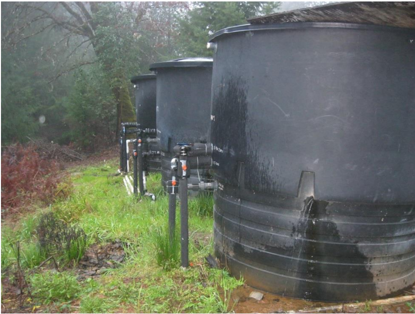
Photo 13 – (3) 3,000 gallon storage tanks.
