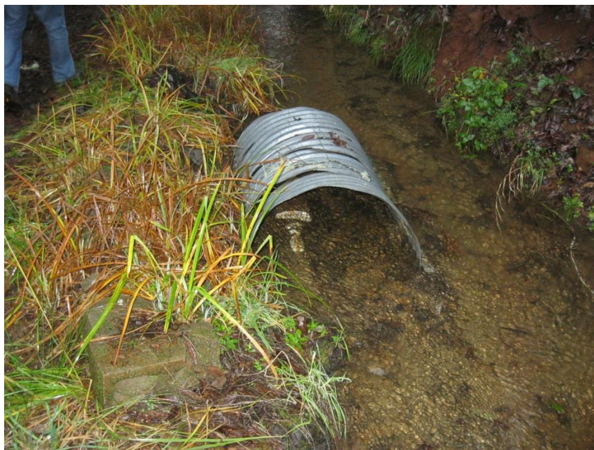
Photo 12 – Intake for water treatment facility.
