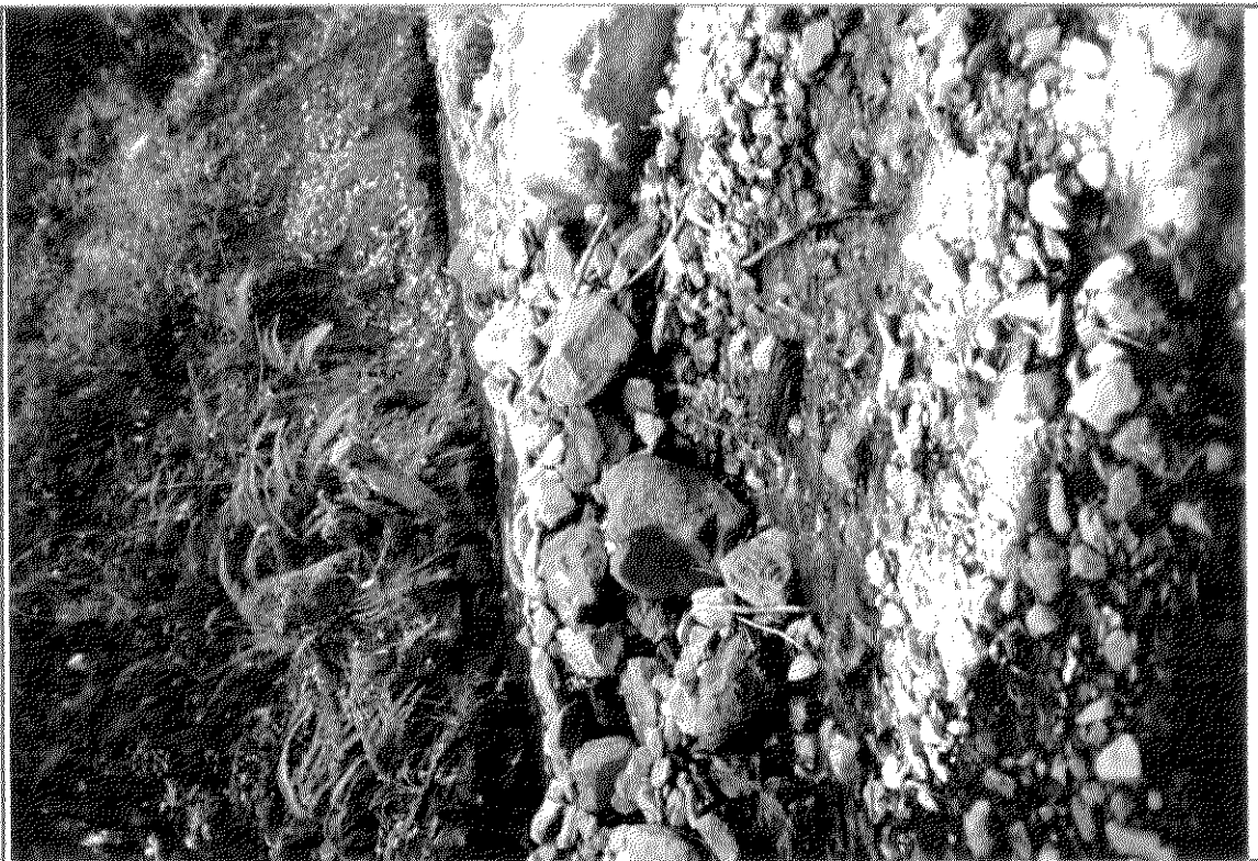
Photo 16. The diversion ditch (top) and water seeping through the “diversion rocks”. The ditch and stream are flowing left to right.
