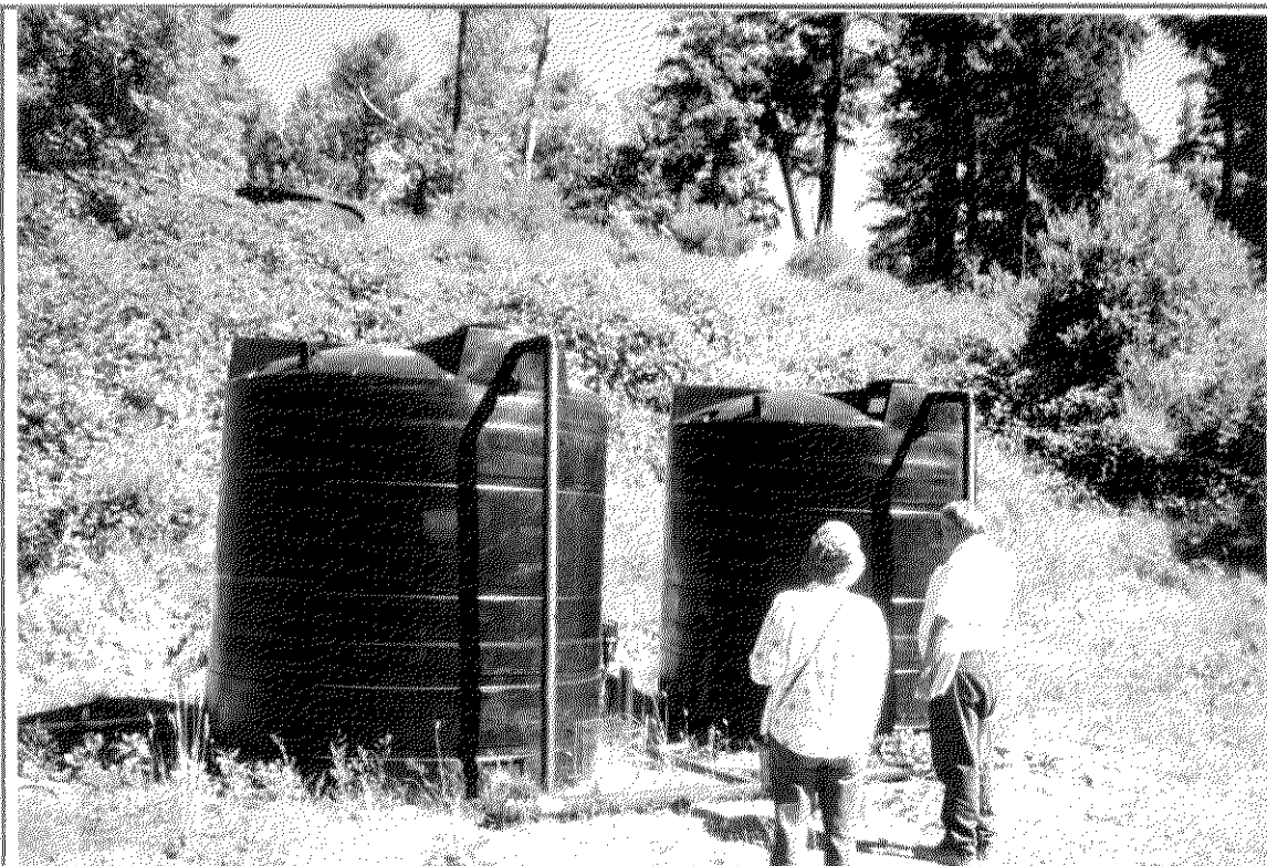
Photo 23. Water purification tanks.
