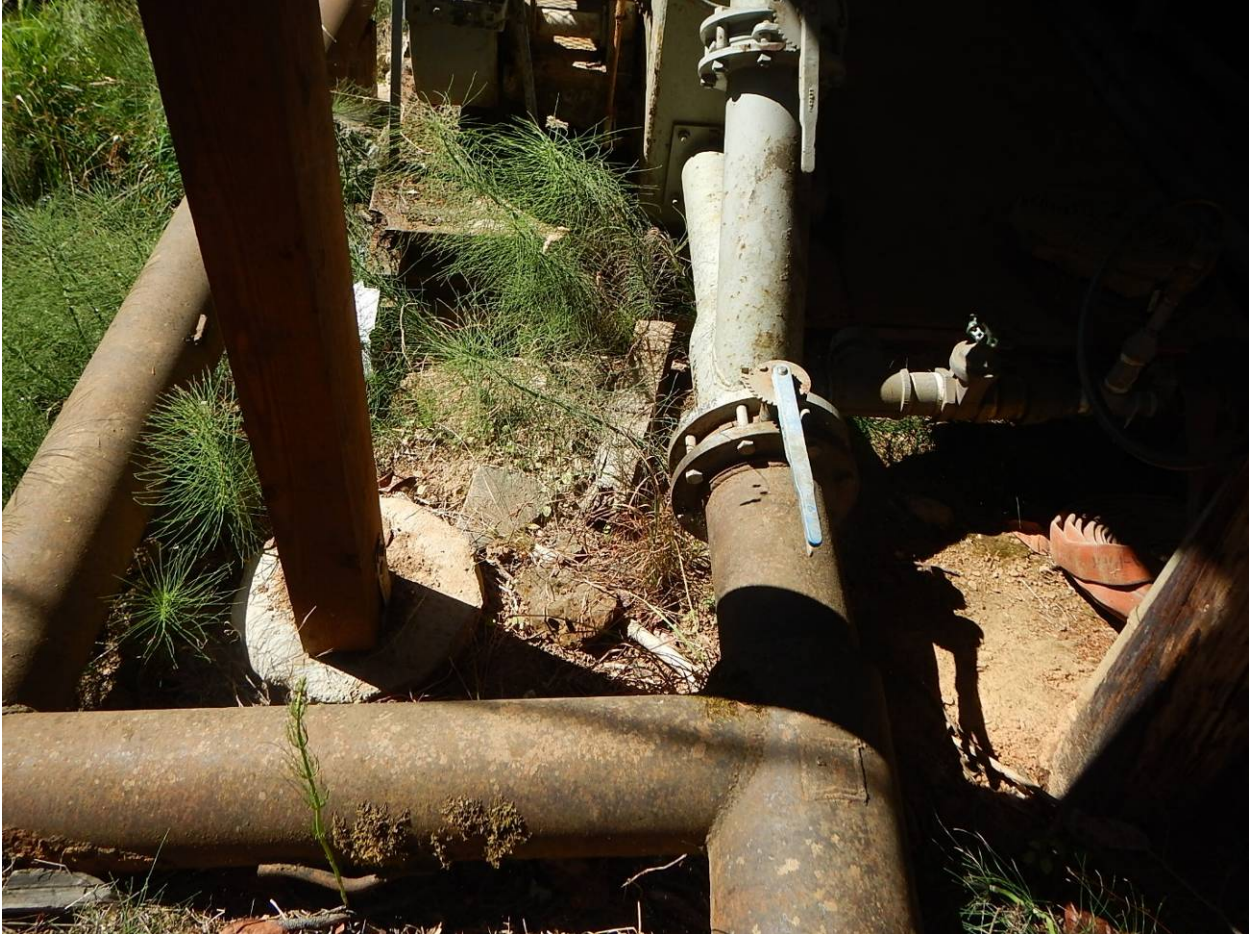
Photograph 6. Junctions near power plant. Tee near the bottom of the photograph serves as junction for flow to power plant and irrigation system. Flow conveyed into the pipe to the left of the photograph serves the irrigation system.
