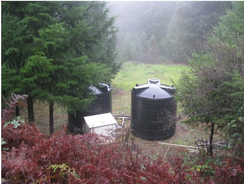
Photo 15 – (2) 3,000 gallon storage tanks.
