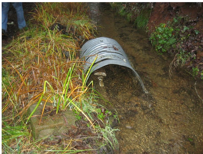
Photo 12 – Intake for water treatment facility.
