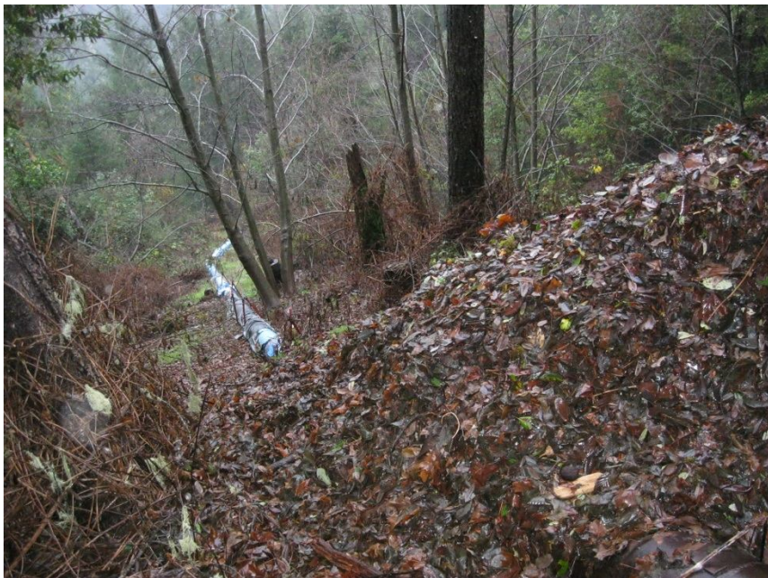
Photo 16 – 14-inch diameter penstock pipe.
