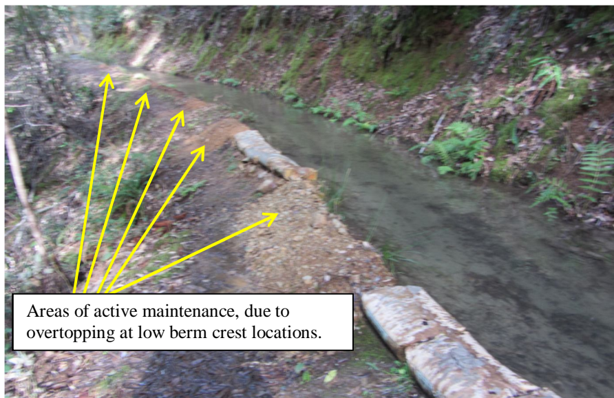
Photo 10 – limited free board space within the ditch.
