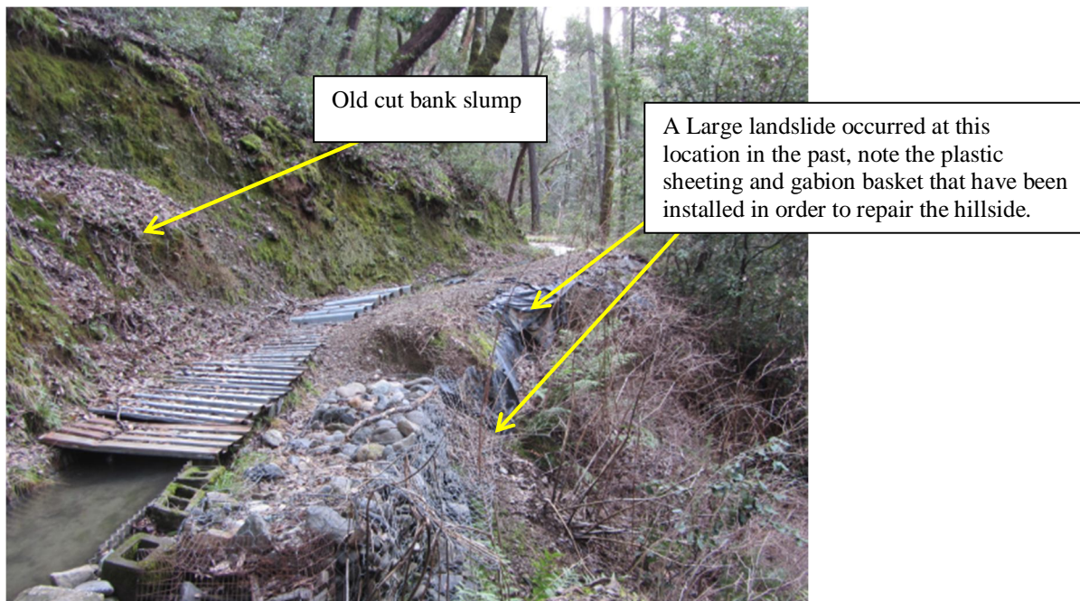
Photo 11 – Large landslide caused by cut bank slump damming ditch and redirecting diverted flow downhill..
