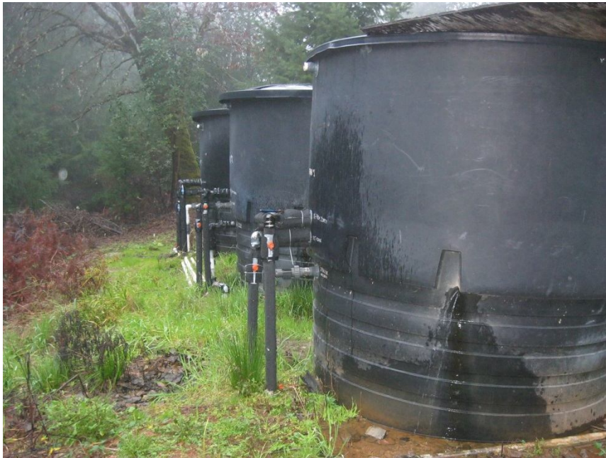
Photo 13 – (3) 3,000 gallon storage tanks.
