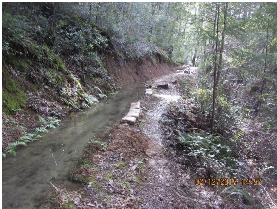
Image 18- Point 12 shows evidence of a recent bank failure that caused water to overtop the outboard berm and erode slopes below the ditch. The outboard ditch shows signs of seepage throughout this length. Note the sand bags and fresh soils along the outboard berm, indicating recent repairs. Also, note the 50-75 foot section of the cut bank with exposed soils. (Photo 8503)
