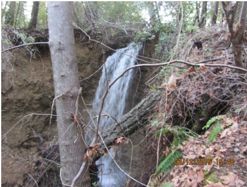
Image 26- Point 20 is the headcut upslope from Irving Creek. This is where tailwater from the Stanshaw Diversion is discharged to an unnamed stream, tributary to Irving Creek. This area is actively eroding. Several trees appear to have fallen recently through erosion of their root masses. I estimate that the headcut erosion has delivered between 1500-2200 yds 3 of sediment to the Irving Creek watershed. (Photo 8529)
