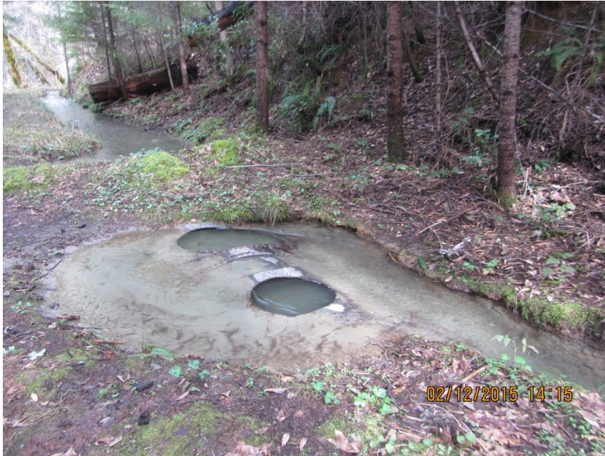
Image 8- at Point 3, shows a closer view of the buried tank car with stored sediments visible. (Photo 8450)
