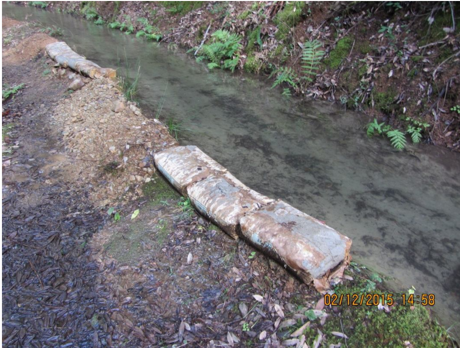
Image 19- Point 12, closer view of berm repair made with ready crete concrete sacks and soils. Note the saturated soils along the outboard berm where water is seeping. (Photo 8510)
