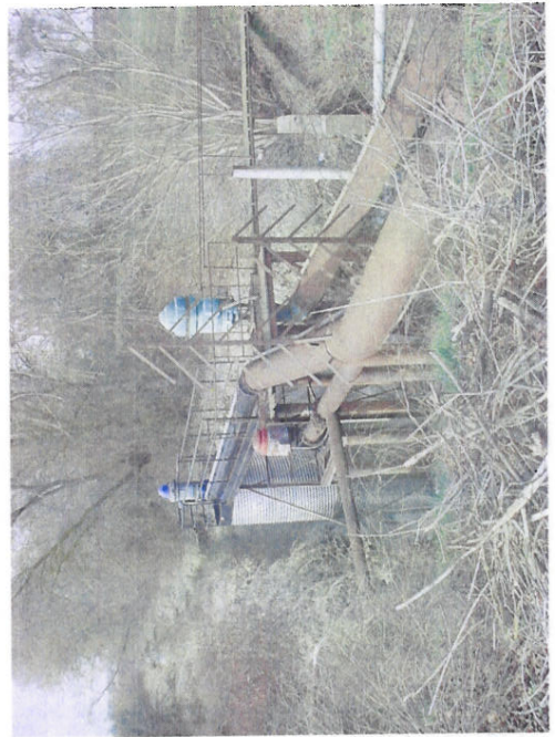
South Pumping Plant and Canal looking west
