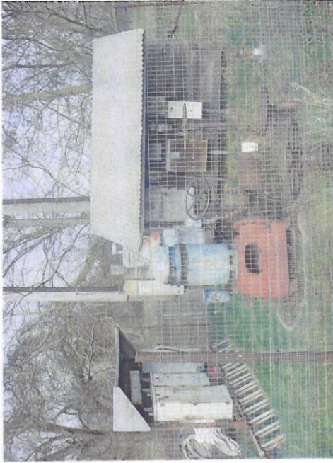
South Pump Electrical Controls and Booster Pumps (40HP & 75 HP)
