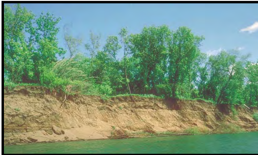
Figure 7: Erosion of the Upper Russian River channel due to incision largely caused by the Coyote Dam. Channel erosion results in direct delivery of fine sediment into the Russian River which is listed as impaired by this pollutant.
