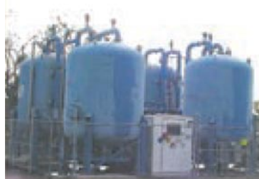
Well-head treatment facilities to remove water contamination.
