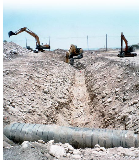
Construction activities such as excavation, grading, and construction vehicles crossing the project sites can be noisy.
