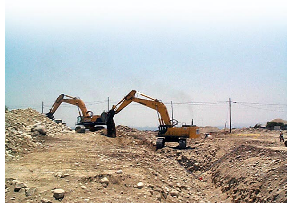
Excavation in the Muni service area, such as the pipeline pictured here, can produce air quality impacts. During excavation and grading, fugitive dust emissions would be released, and construction equipment and vehicles would generate emissions.
