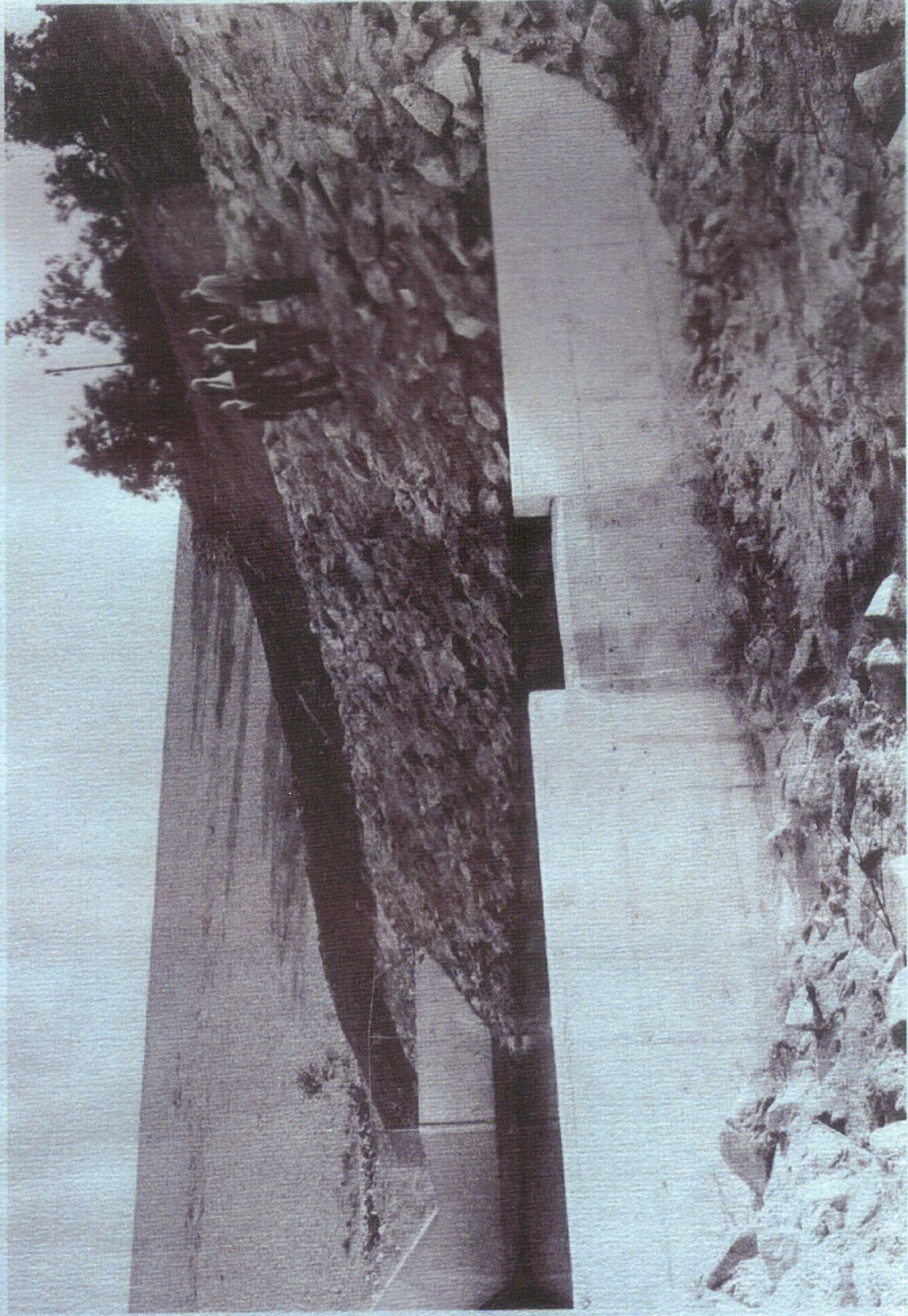
Completed Restoration of Outlet Works at Villa Park Dam. Inspecting Officials Stand on Grouted Riprap Sidewall. Staff.
