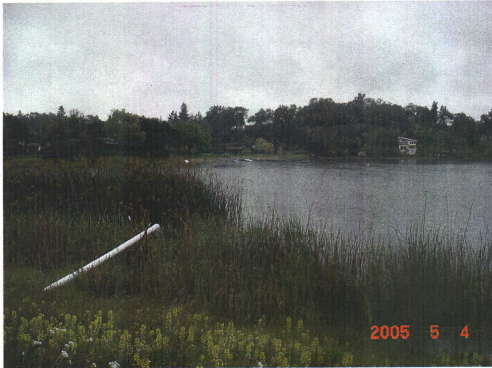
This photograph shows the outlet of the diversion pipe at the reservoir.
