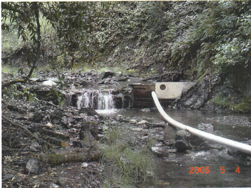
Diversion dam and 4-inch PVC pipe at the point of diversion to offstream storage.
