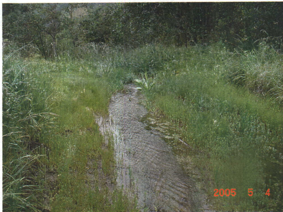
View of flow out the spillway looking downstream. The flow was not measured but appeared to be less than the inflow from the diversion pipe.
