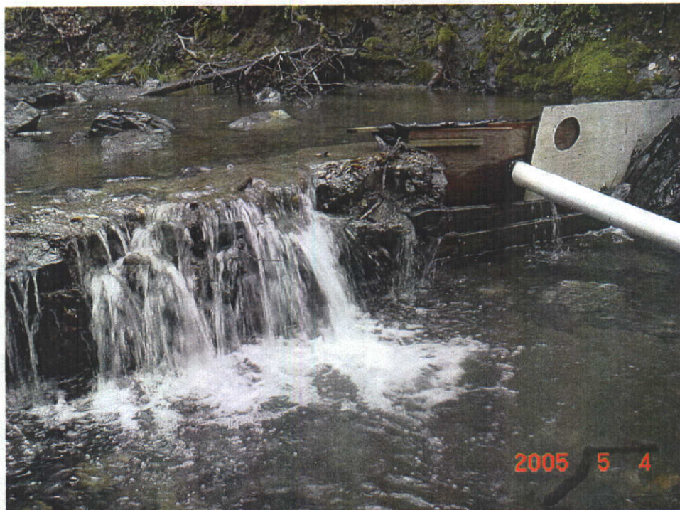
There was no measuring device at the point of diversion to verify the bypass. The gap in the diversion dam is filled with wood scraps that appear to include the original measuring device.
