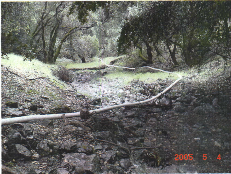
This photograph shows the 4-inch PVC pipe in the streambed immediately below the POD.
