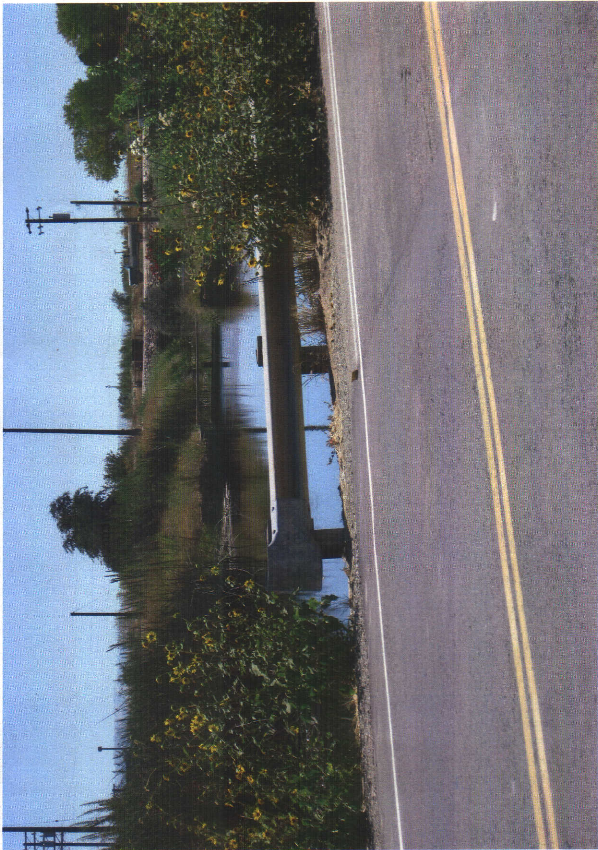
Woods Irrigation Company West Main Canal at Howard Road Looking southerly and upstream toward the Point of Diversion
