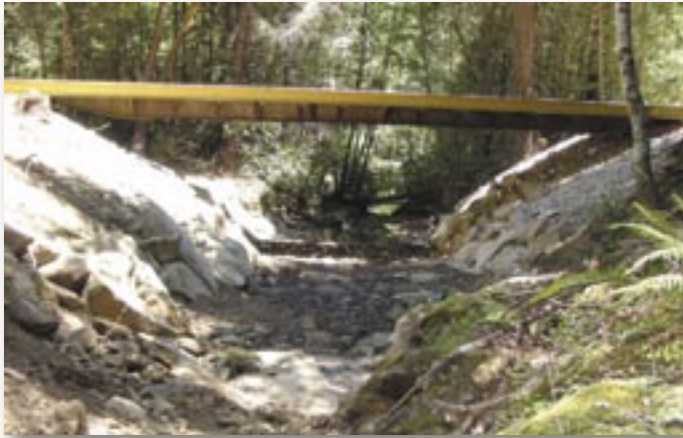
Before and After: Little Waldron Creek Fish Passage Barrier Replacement in Mendocino County.
