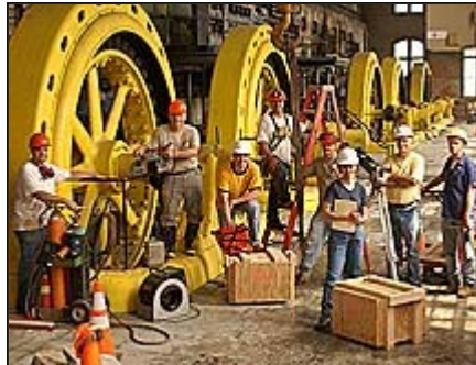
Preparations begin for rehabilitation of the Mechanicville Hydroelectric Project, Mechanicville, NY (photo Fourth Branch Associates)
