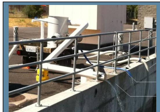
Organic Matter Separation Test Unit at A-Canal Fish Screen
