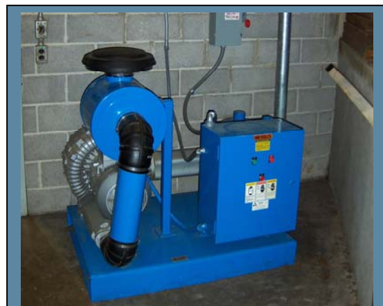
Turbine Venting Blower at Iron Gate Dam
