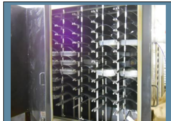
New Moist-Air Incubators at Iron Gate Hatchery
