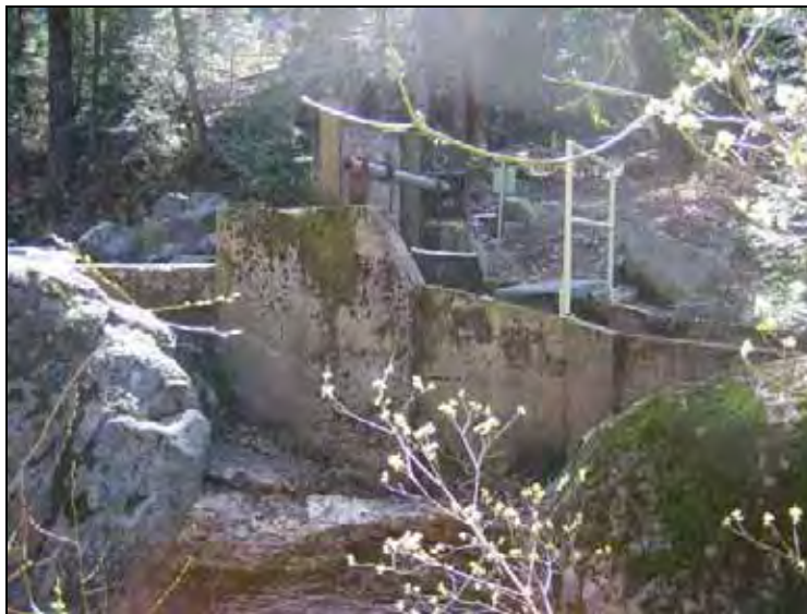
Feature 1: Kilarc Main Diversion, Gate and Gate Operator. Facing: Southeast (Photo acc. # 482-12-1-30)
