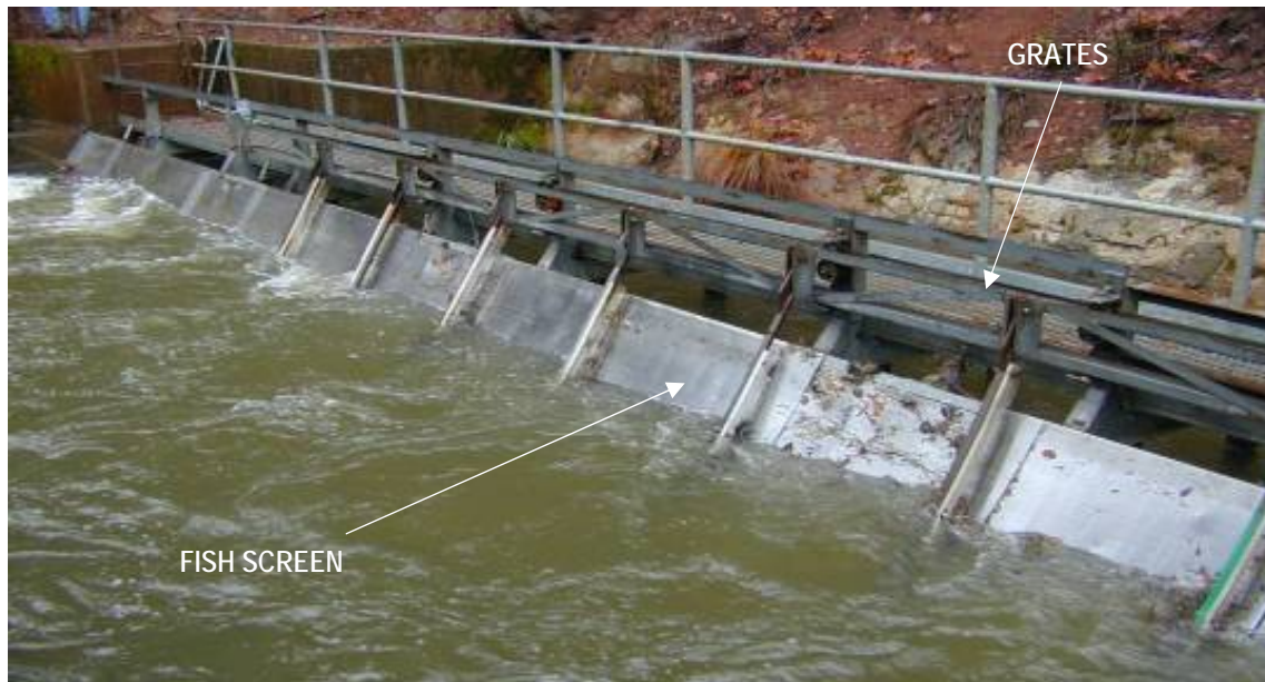
Photograph 2.3.3-1c South Cow Creek Diversion – Fish Screen Detail
