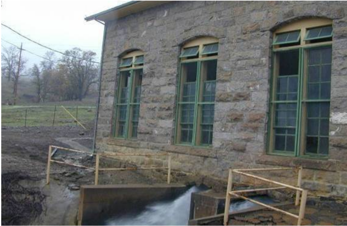
Photograph 2.3.8-1b Cow Creek Powerhouse
