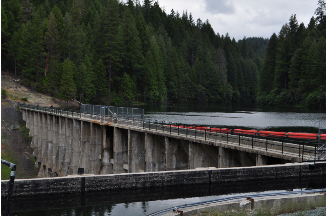
Key View 5. View from near the existing spillway structure looking north toward the dam and reservoir.
